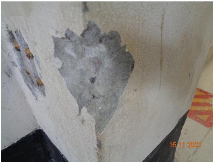
Stone Chips (Compressor & Boiler)
