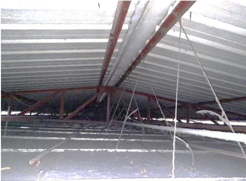
No roof bracing
