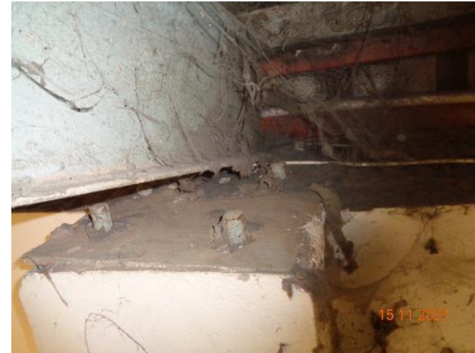
Poor connection details
