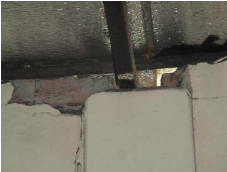
Poor and non-engineered connection
