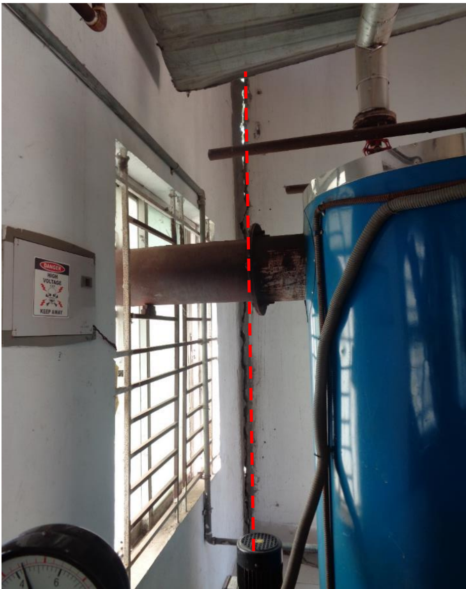
Brick wall drifted (apparently) from original position
