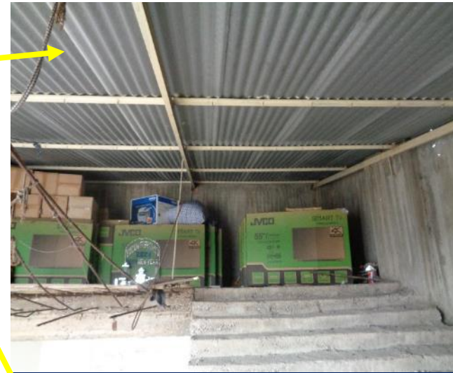
No apparent load path with poor connection
