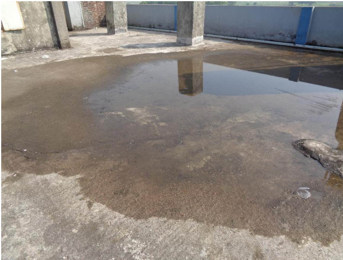
Water ponding on roof slab due to poor drainage system
