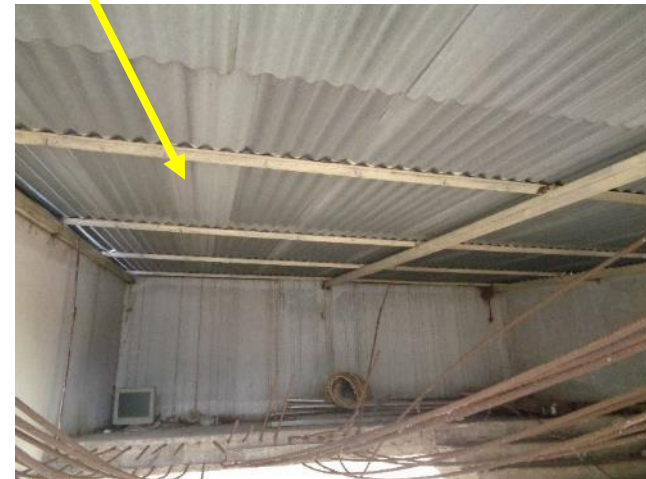
No apparent load path with poor connection
