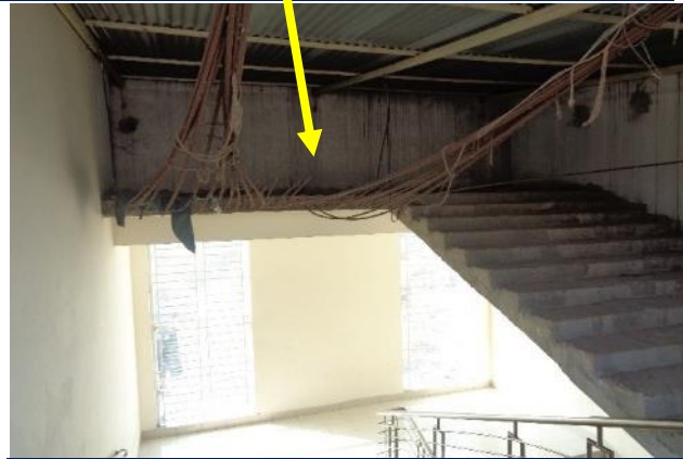
No apparent load path with poor connection
