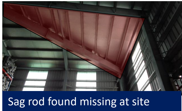
Sag rod found missing at site
