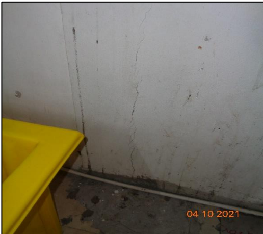
Cracks on internal brick wall
