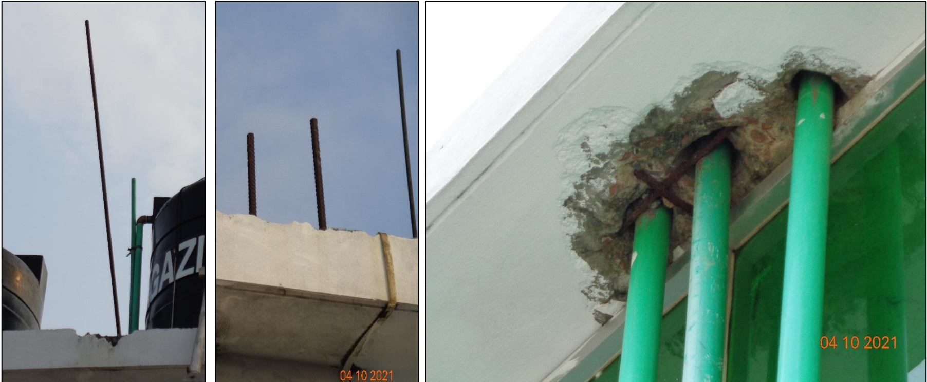
Exposed rebar at roof
