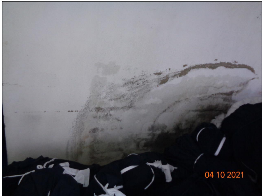
Dampness on brick wall
