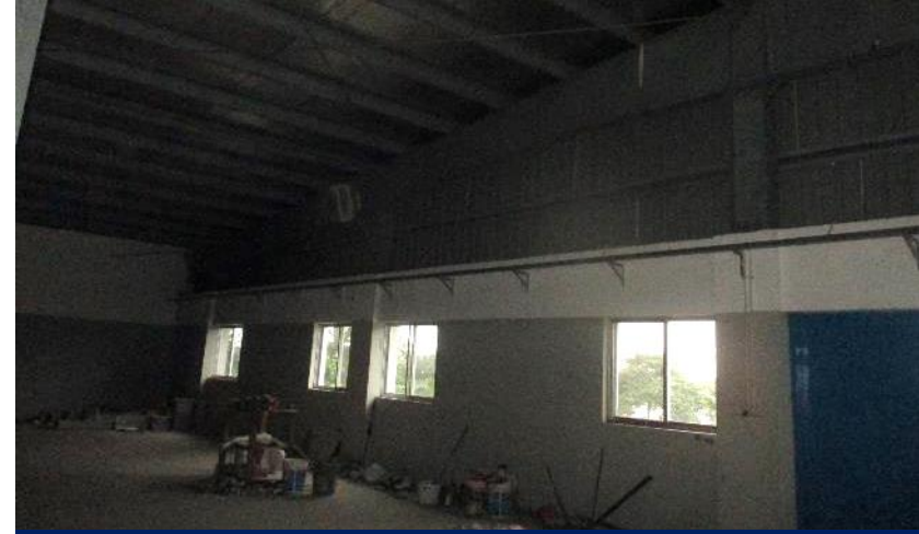
No load plan was prepared for mezzanine floor
