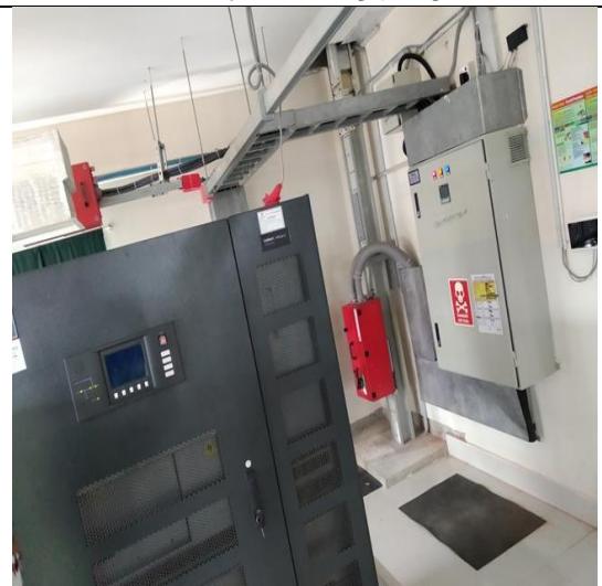
Typical cable entry system into electrical panel in production floors.
