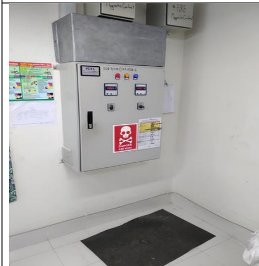
Typical electrical distribution panel.
