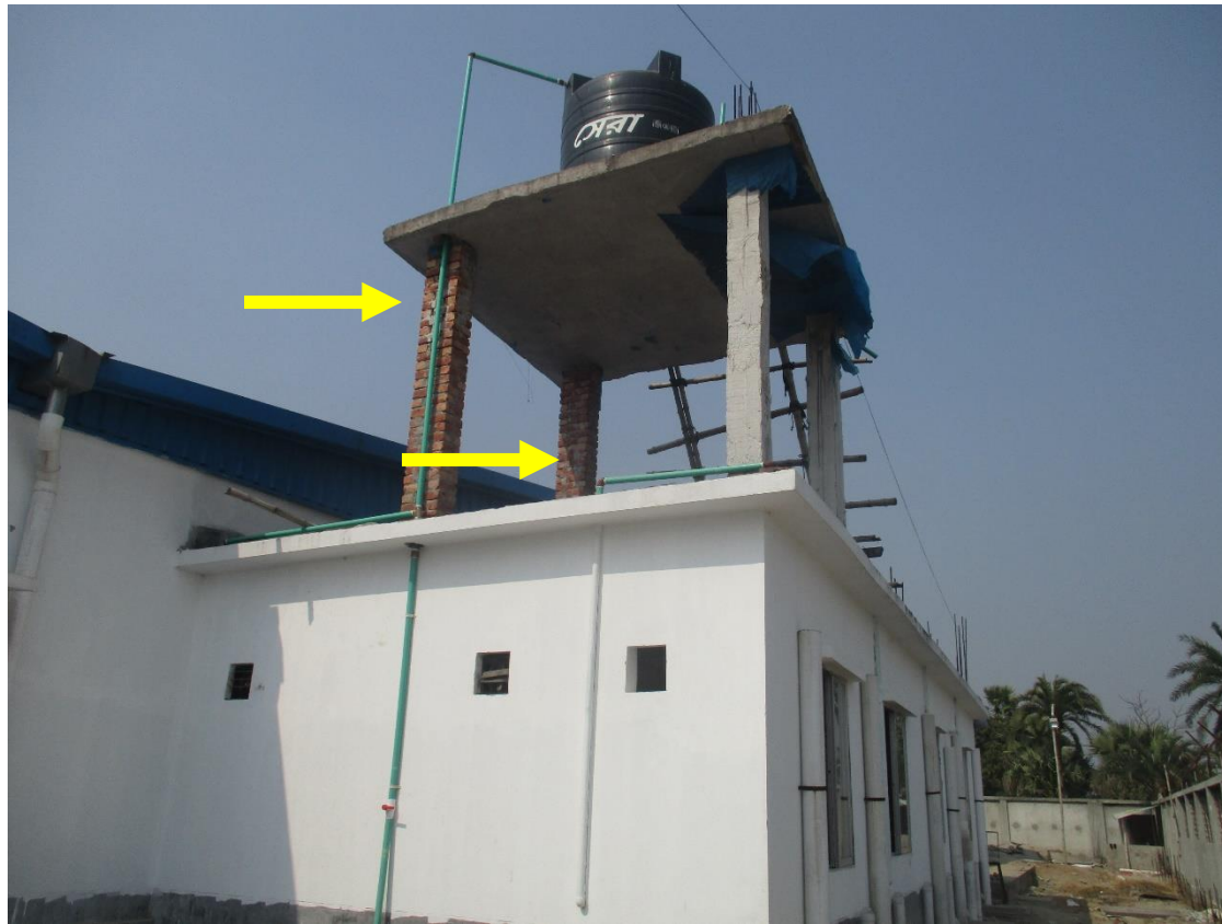
Water tank supported on unstable platform
