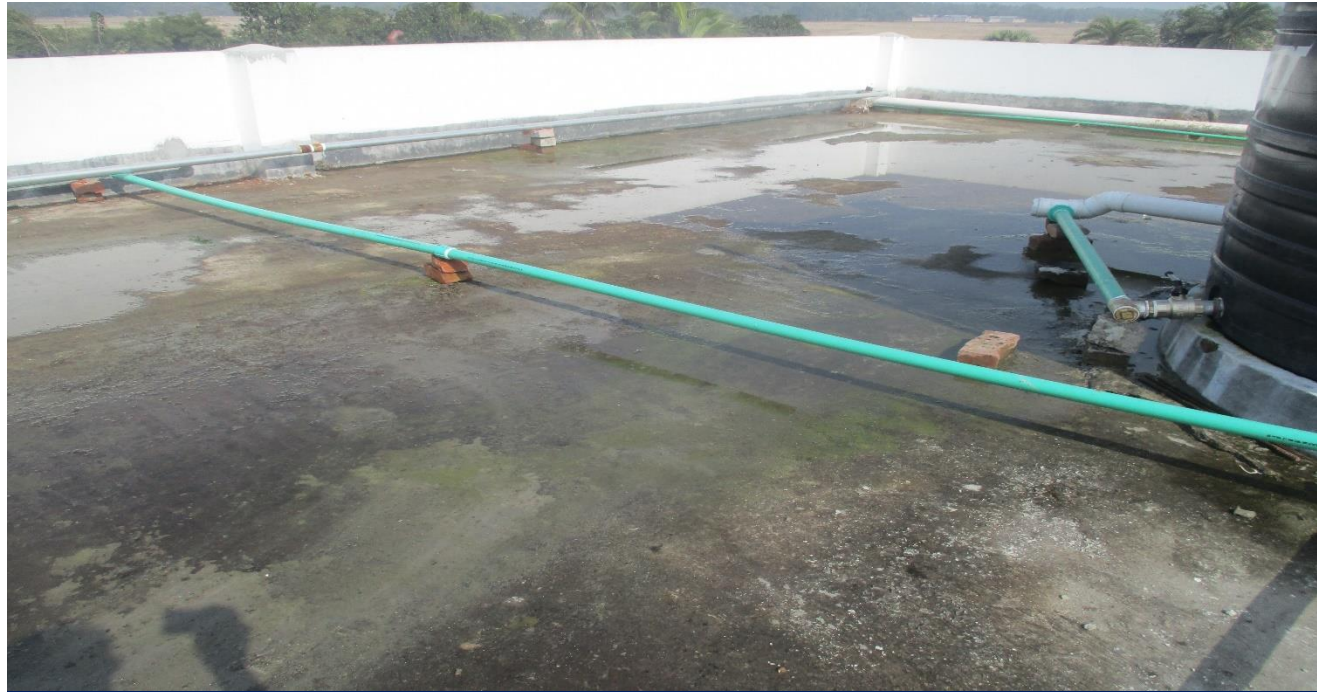
Water ponding on roof slab at Building-1
