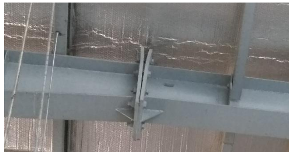
Gap between rafter-rafter connections
