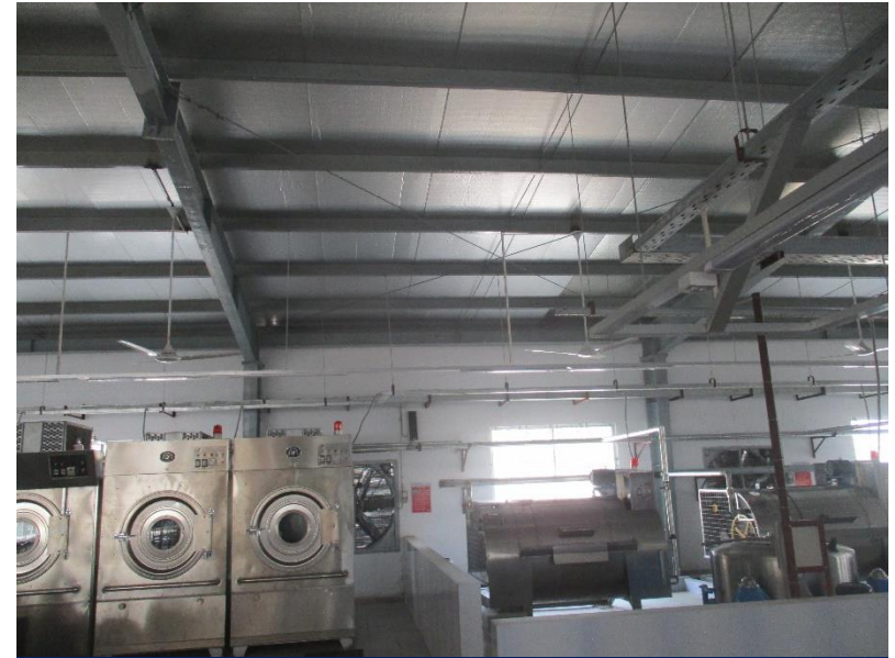
Loose roof bracing
