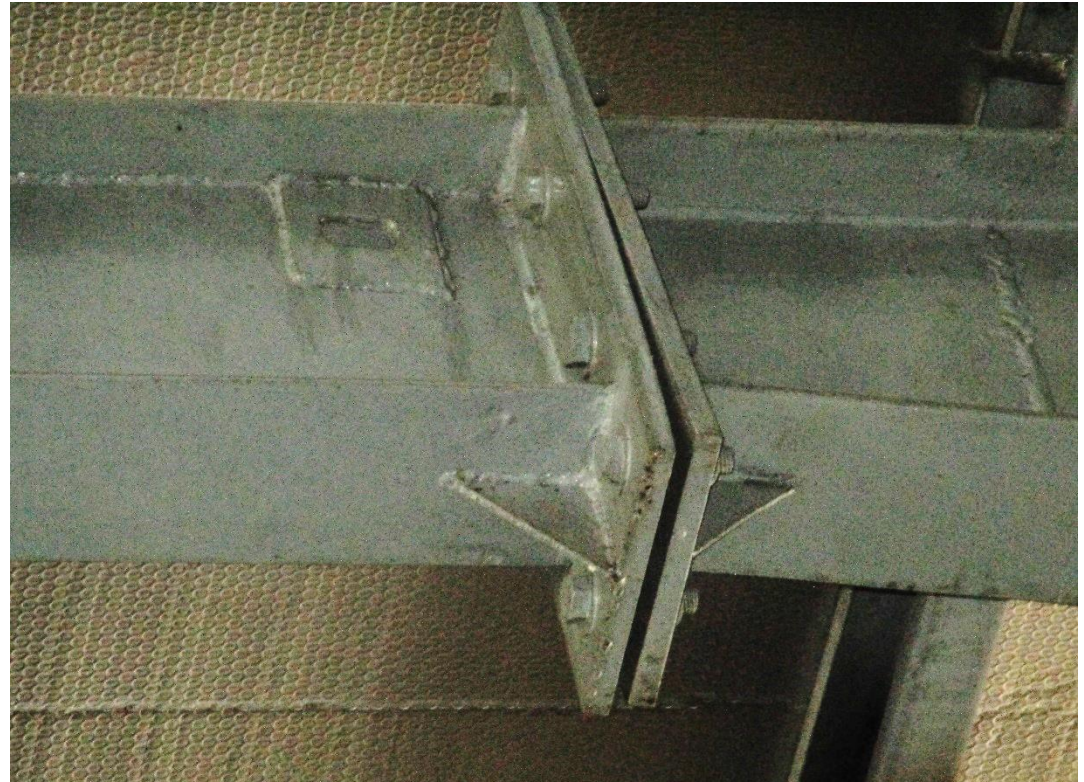
Gap between rafter-rafter connections
