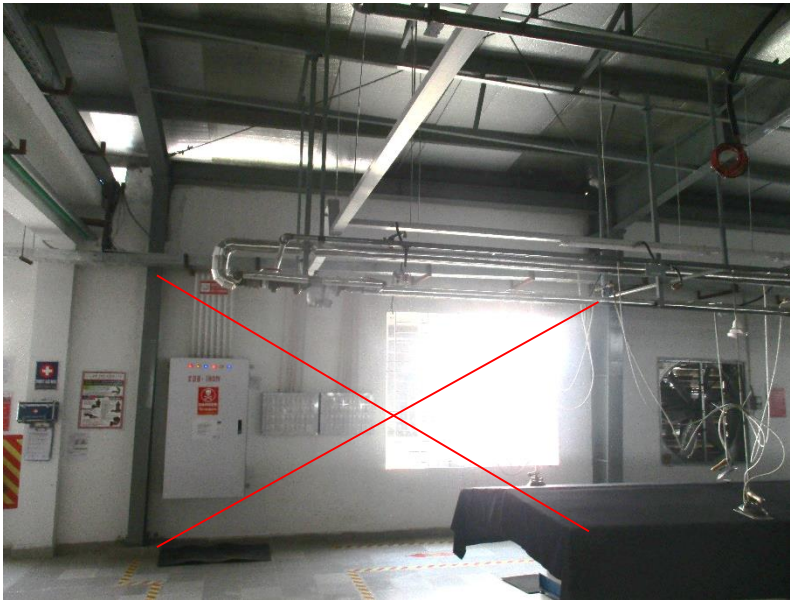
Missing vertical bracing
