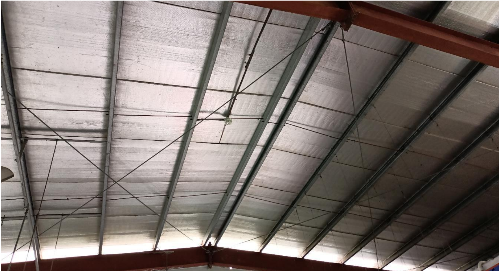
Loose cable bracing at roof
