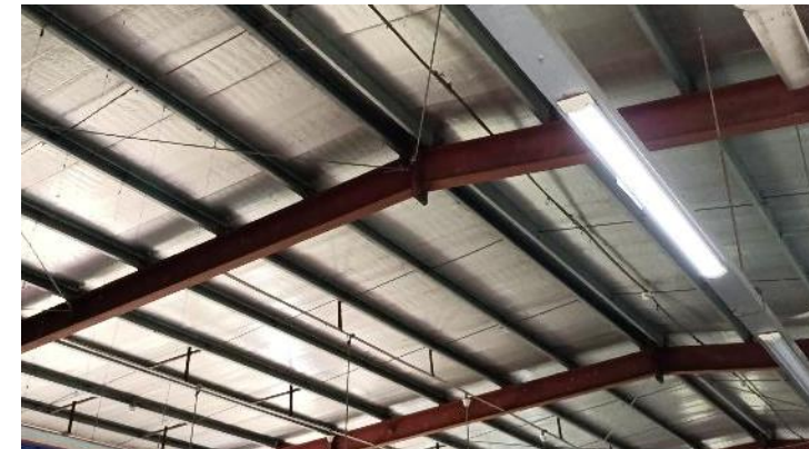
No flange bracing onsite
