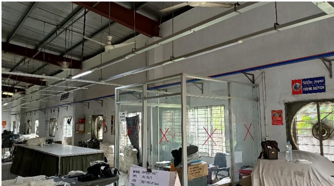
No vertical Bracings on site
