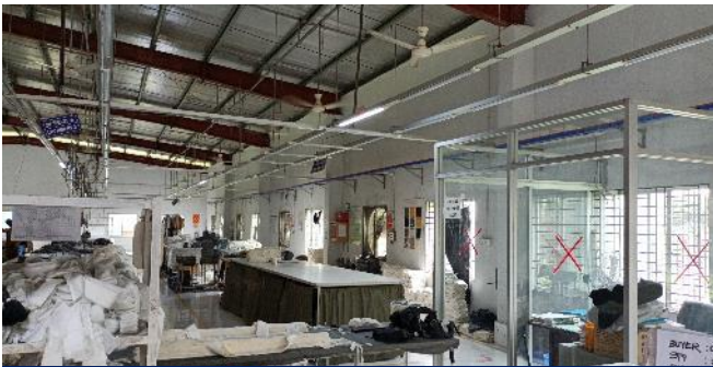
No vertical Bracings
