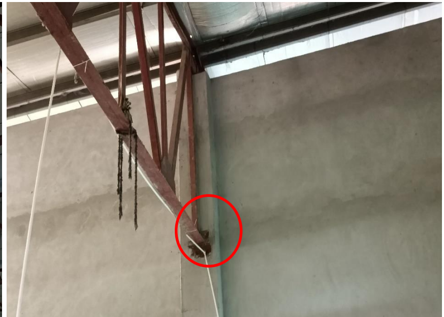
No connection details found for seat connection at grid-7
