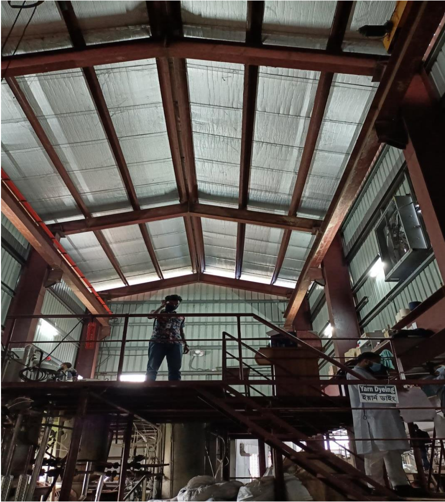
No roof bracing
