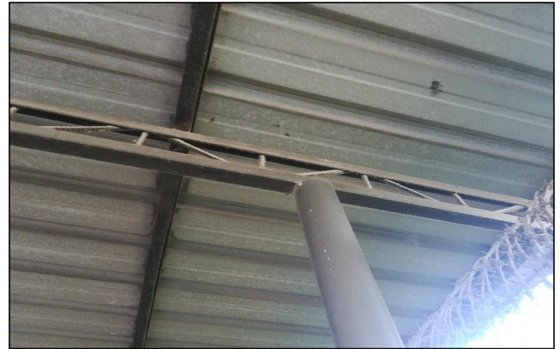
Poor connection details (Shed-6)
