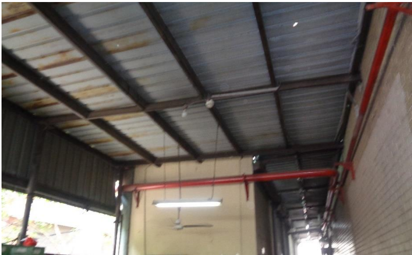
Inadequate structural members (Shed-5)
