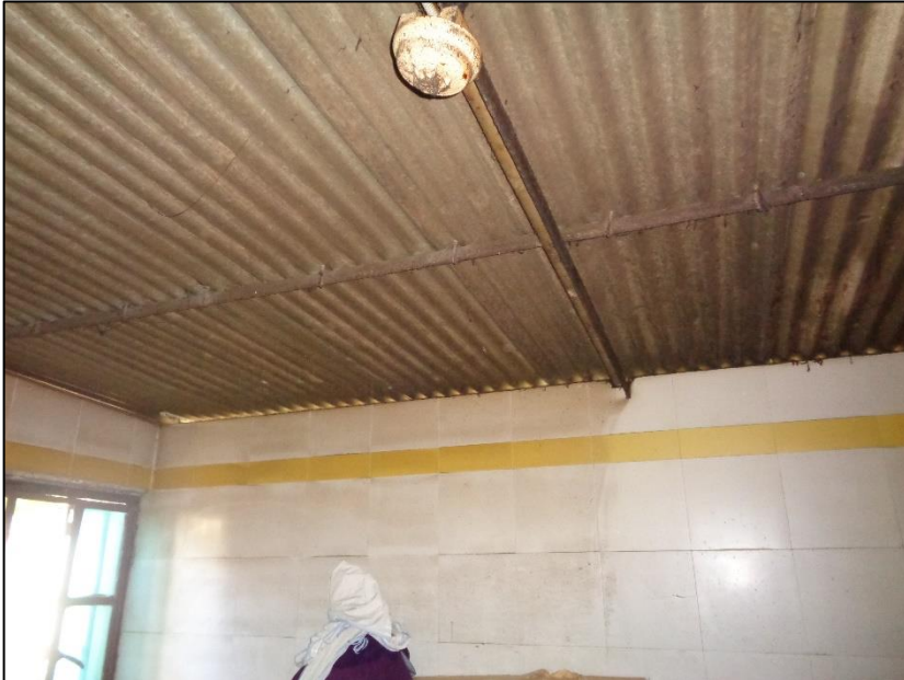
Inadequate structural members (Shed-11)
