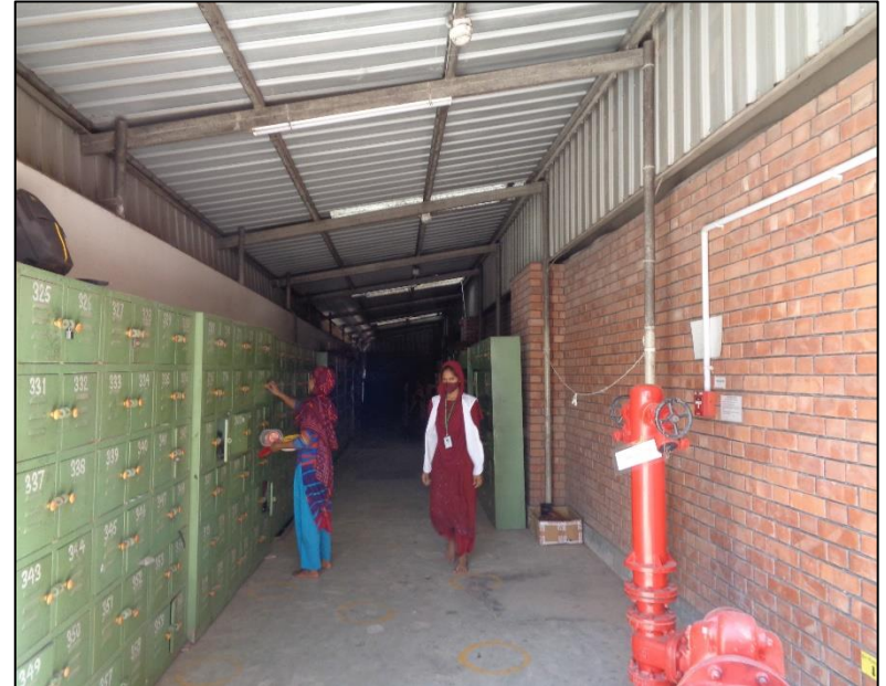
Inadequate structural members (Shed-12)
