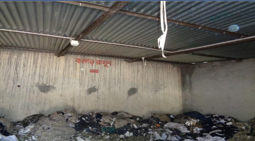
Inadequate structural members (Shed-7)
