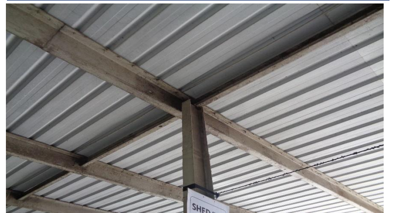
Poor connection details (Shed-10)
