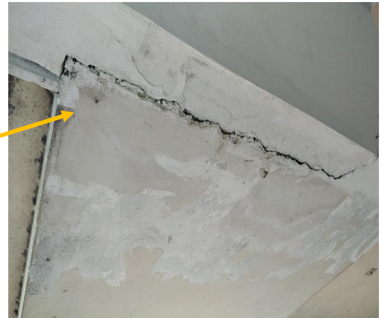
Crack of drop wall
