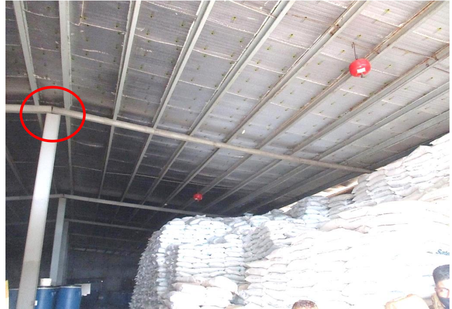
No bracing system; Rafter deflection at roof level in Part-A
