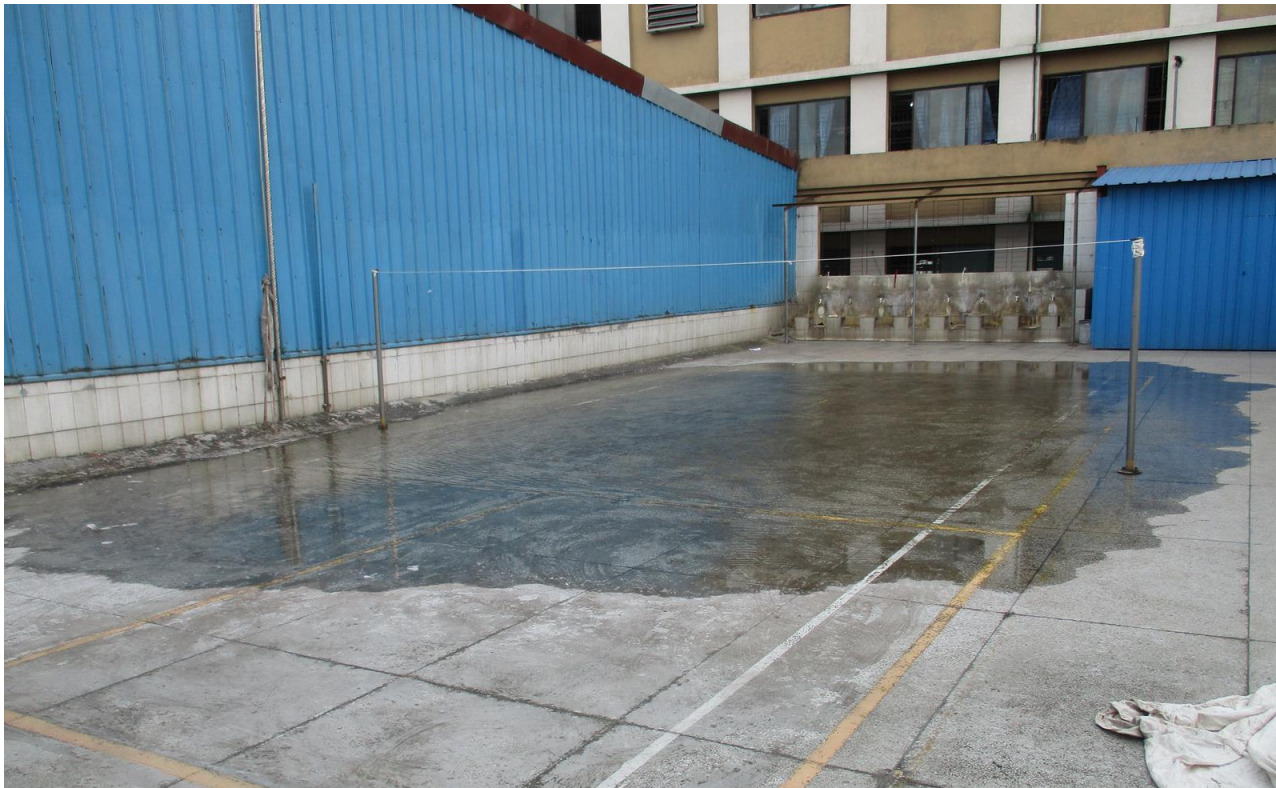
Stagnant water on the open roof area.
