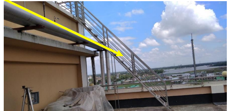
Undocumented steel stair
