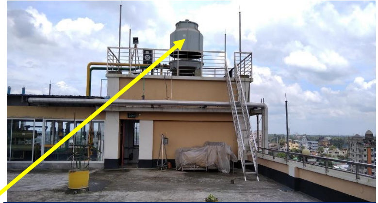
Chiller machine and stair not mentioned in the drawing
