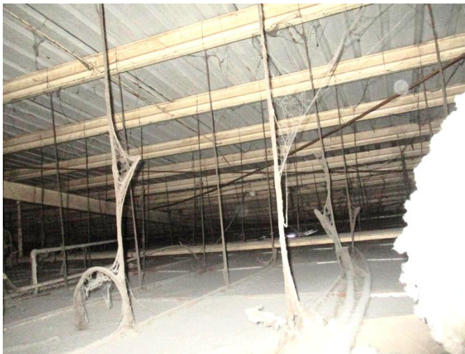
Cable bracing at roof
