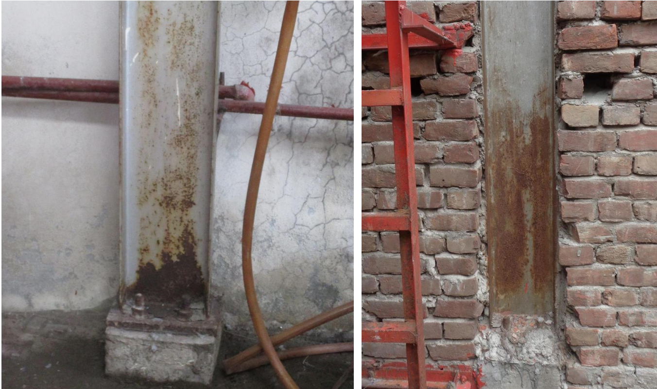
Corrosion on steel member.
