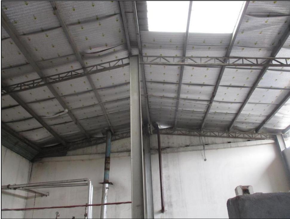
No bracing system at roof
