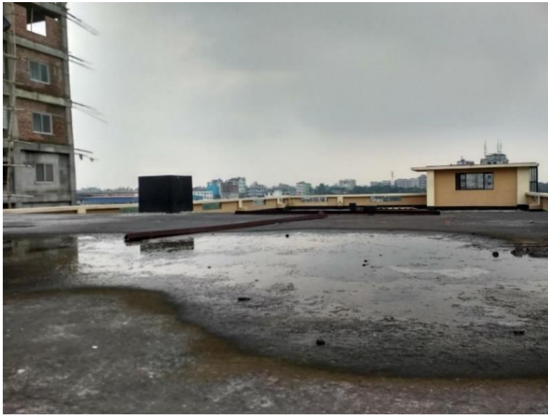
Water ponding on roof
