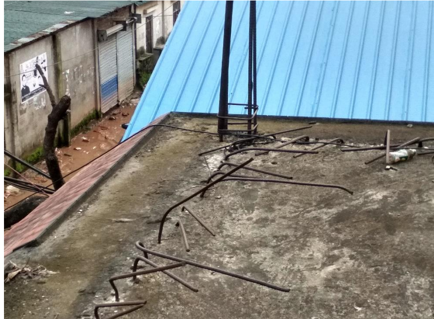
No parapet wall in some area of the roof
