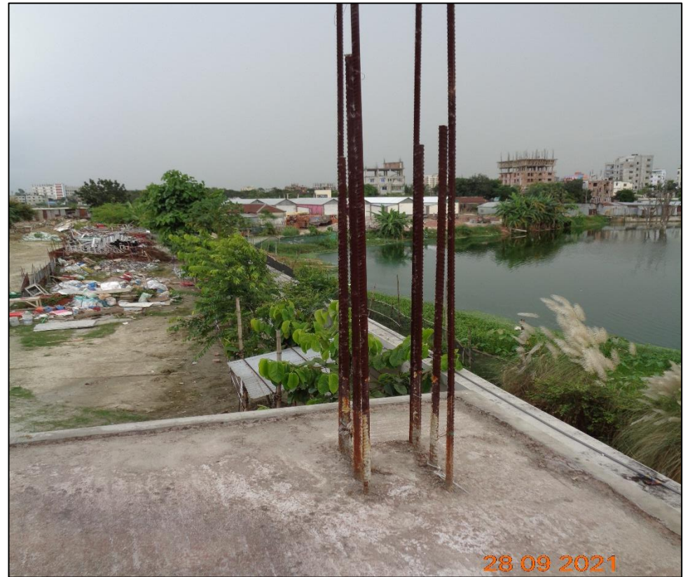
Exposed rebar of Column
