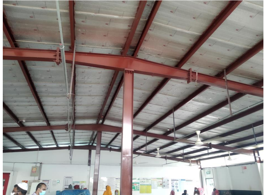
No bracing at roof and wall
