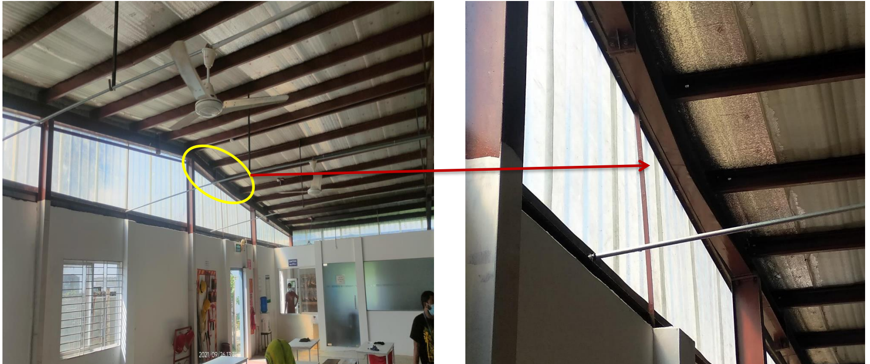
Distorted structural member
