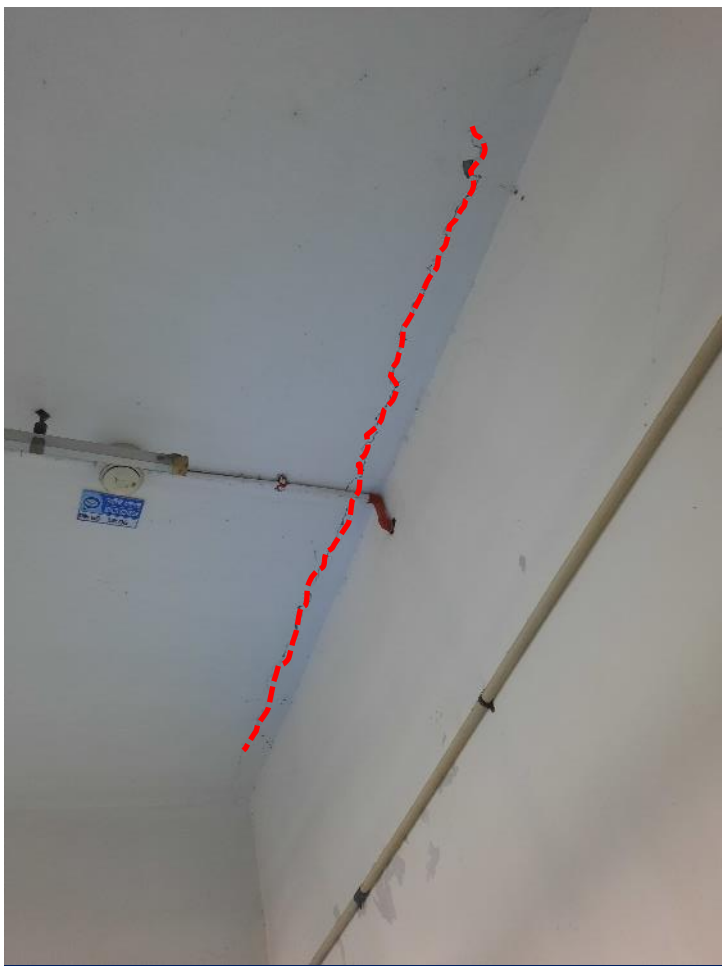
Crack on 1 st floor Slab Soffit
