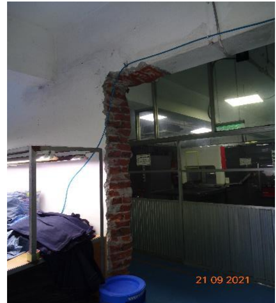
Overhang brick wall without lintel
