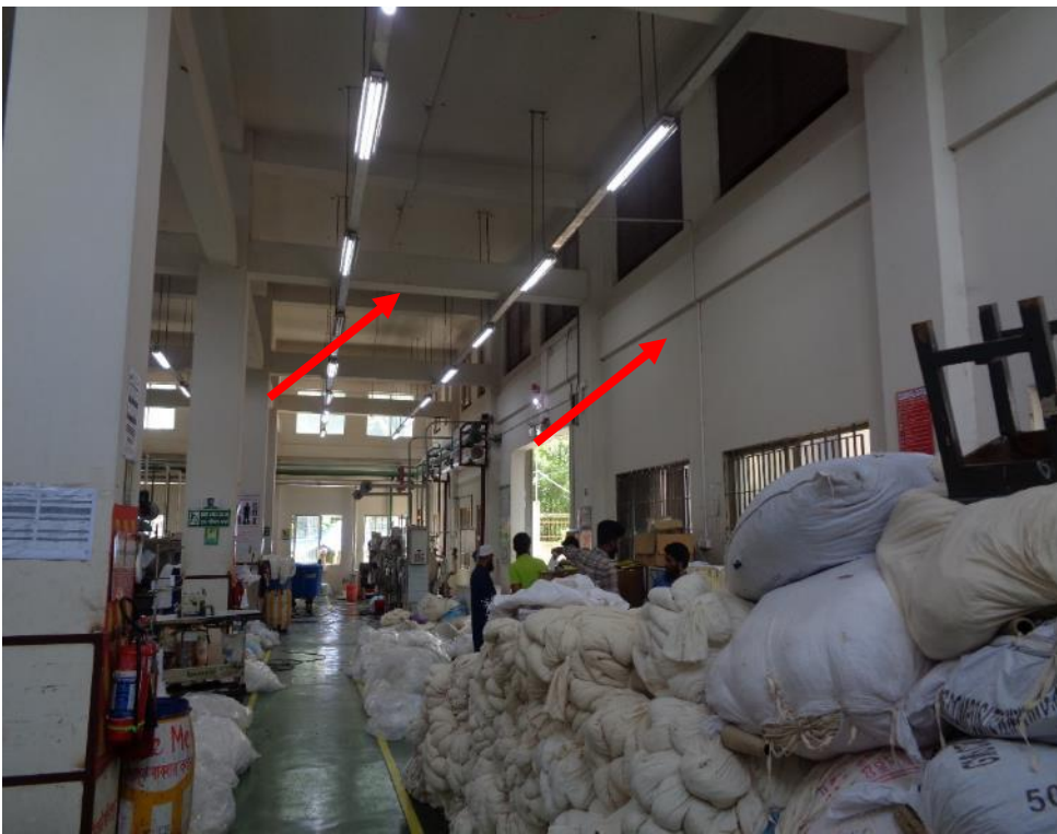
Tie beam of Ground floor found at different levels
