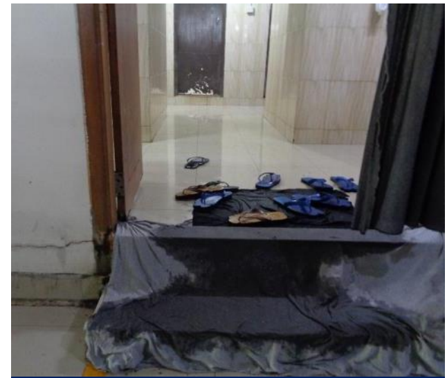
250mm Build up at toilet area
