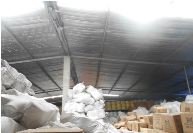
Inadequate structural member
