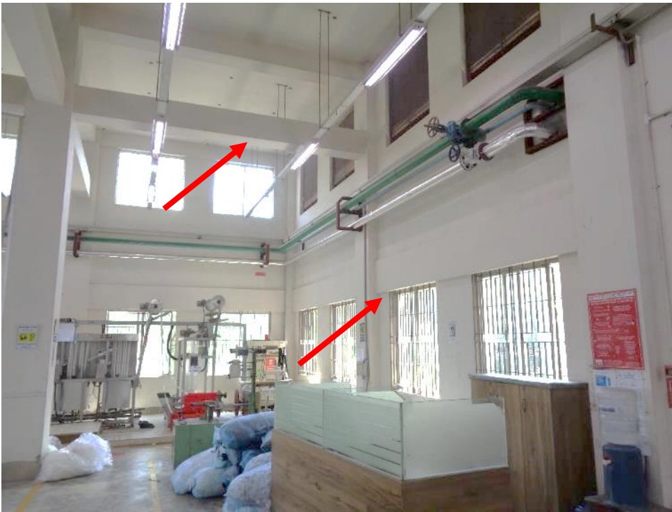
Tie beam of 1 st floor found at different levels
