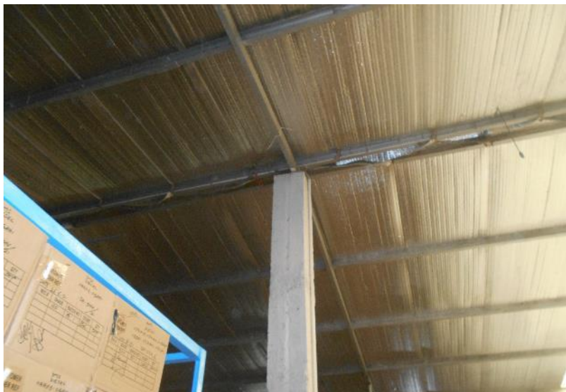
Lack of lateral stability system
