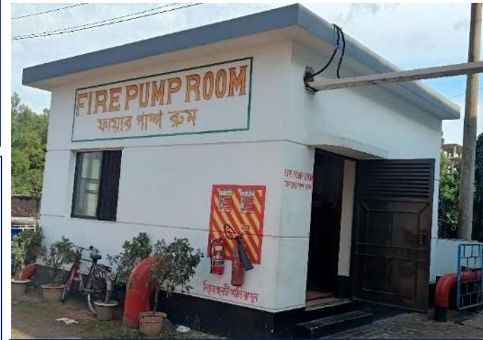
01 No Fire Pump
