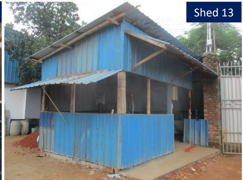
Inadequate structural members
