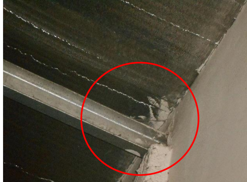
Poor connection details
