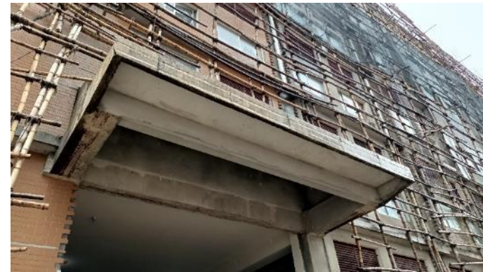
Undocumented Porch at Exits
