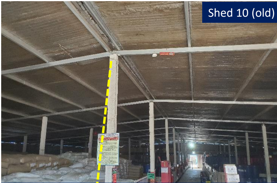
Inadequate structural members
