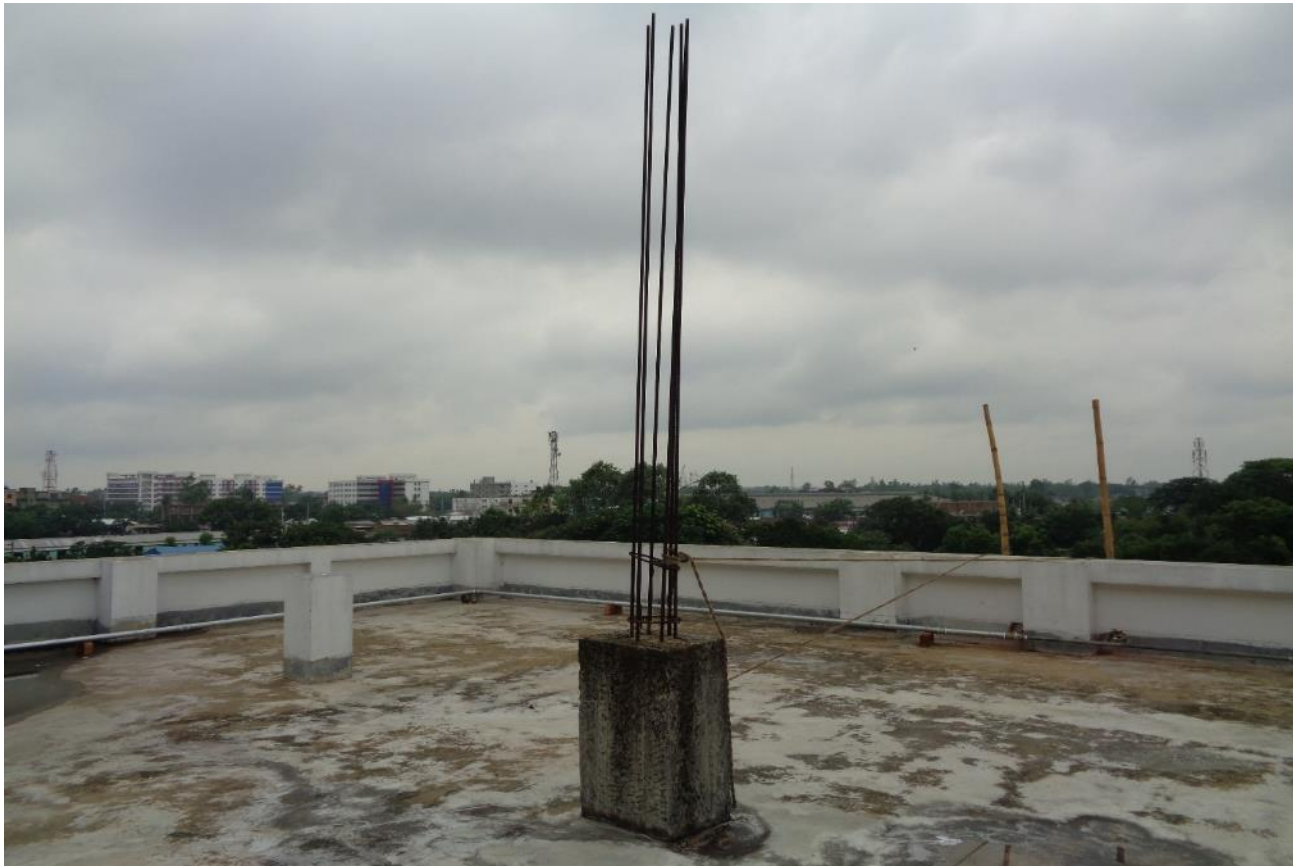
Exposed reinforcement at roof level
