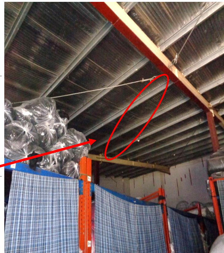
Missing horizontal bracing at roof
