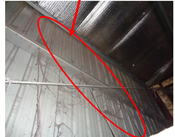
Missing vertical bracing at wall
