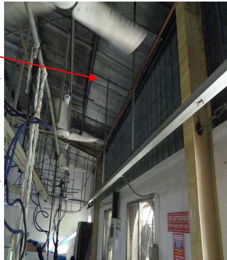
No bracing system
