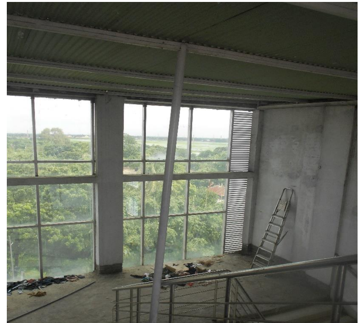
Apparently inadequate member & poor connection details
