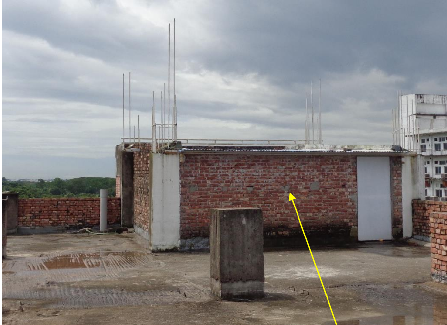
Non-engineered shed over staircases
