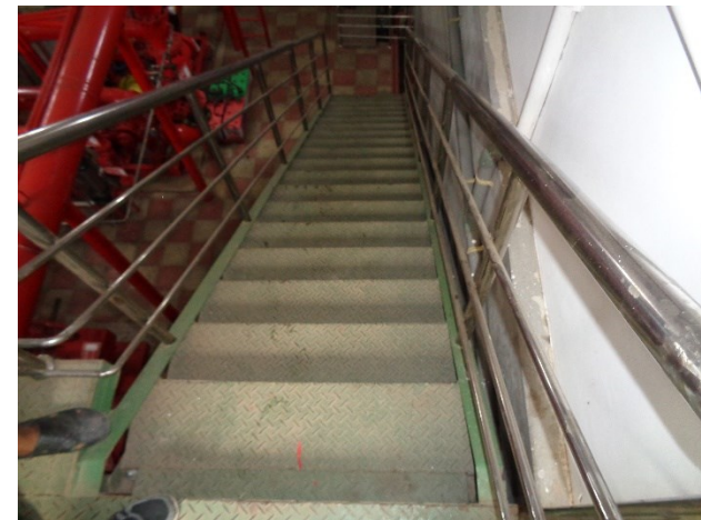
Undocumented steel stair
