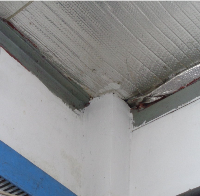
Poor connection details
