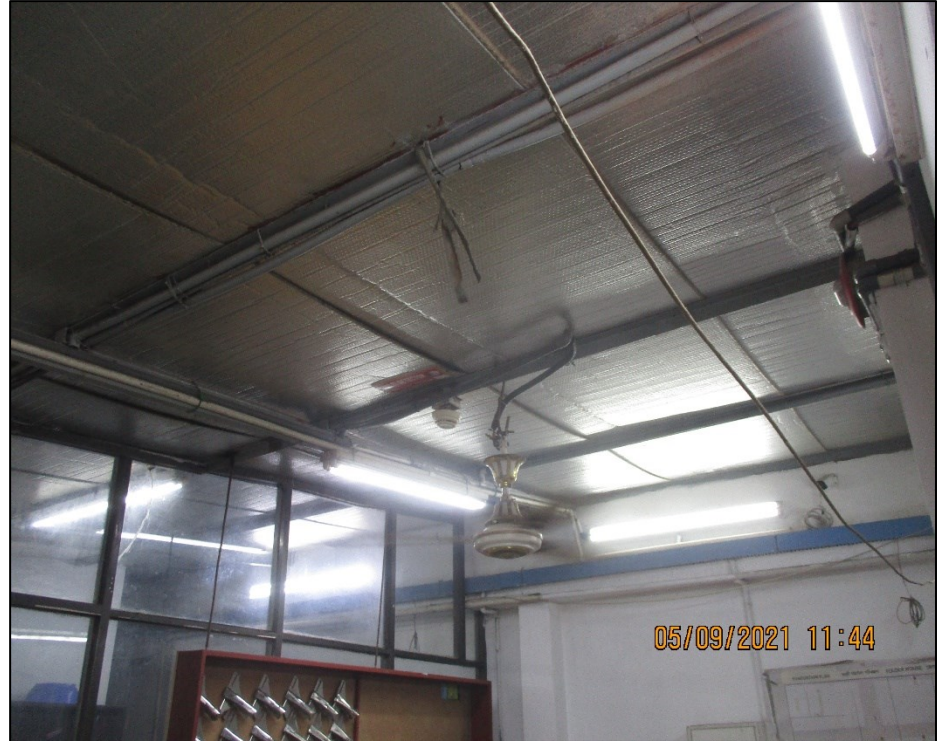
Apparently inadequate structural members
