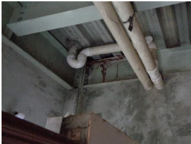
Corrosion in steel beam
