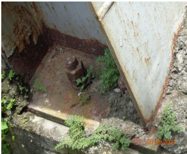
Corrosion in Base Plate
