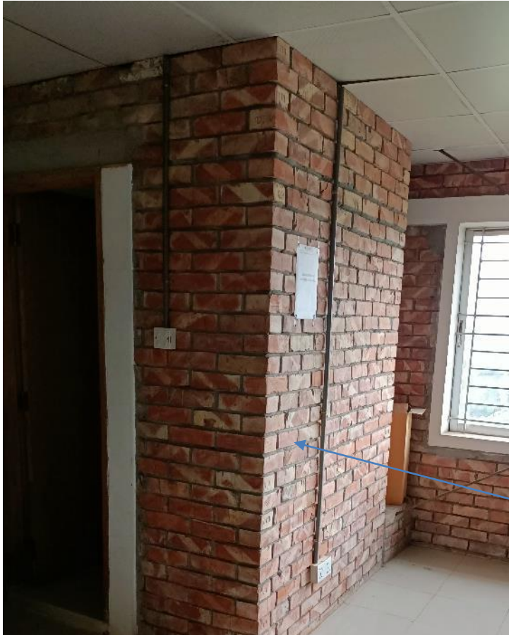
Toilet zone of 1 st floor Not shown in drawings
