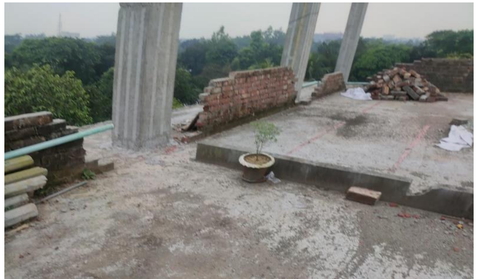
Incomplete parapet wall on the roof
