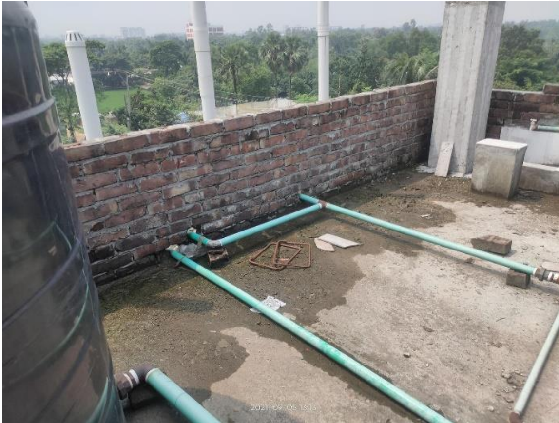
Stagnant water on the roof
