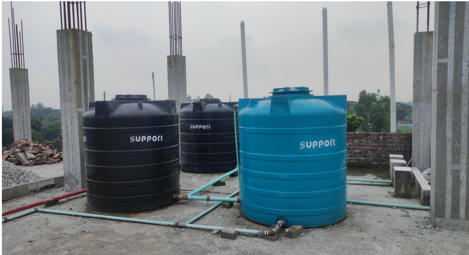
3x2000 liter plastic water tanks on the roof
