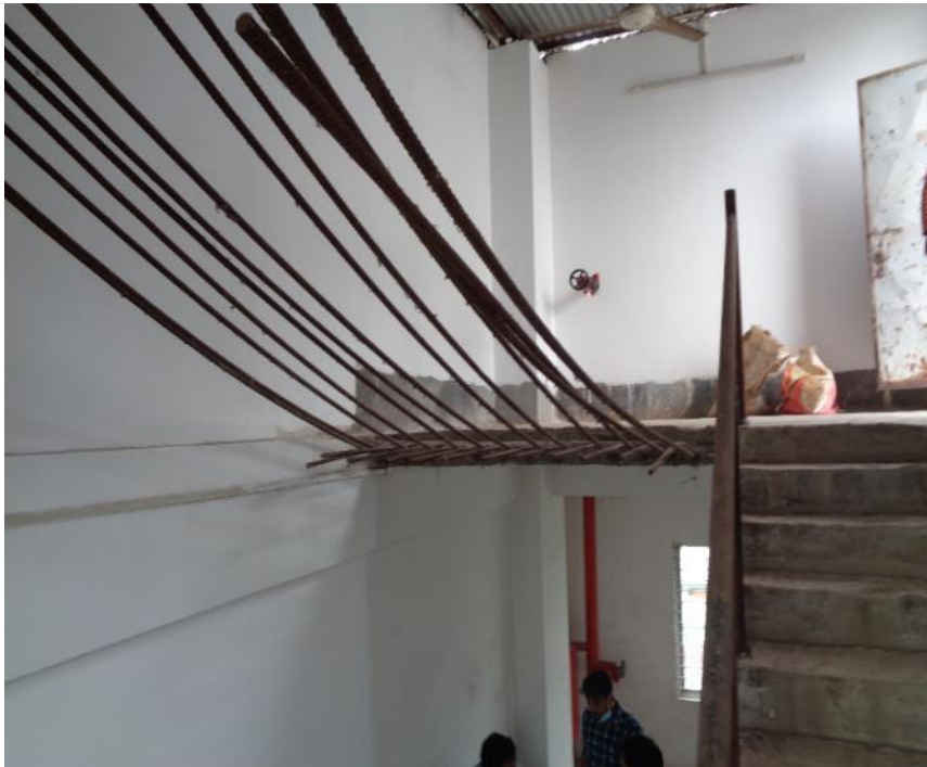
Exposed reinforcement left at Staircase
