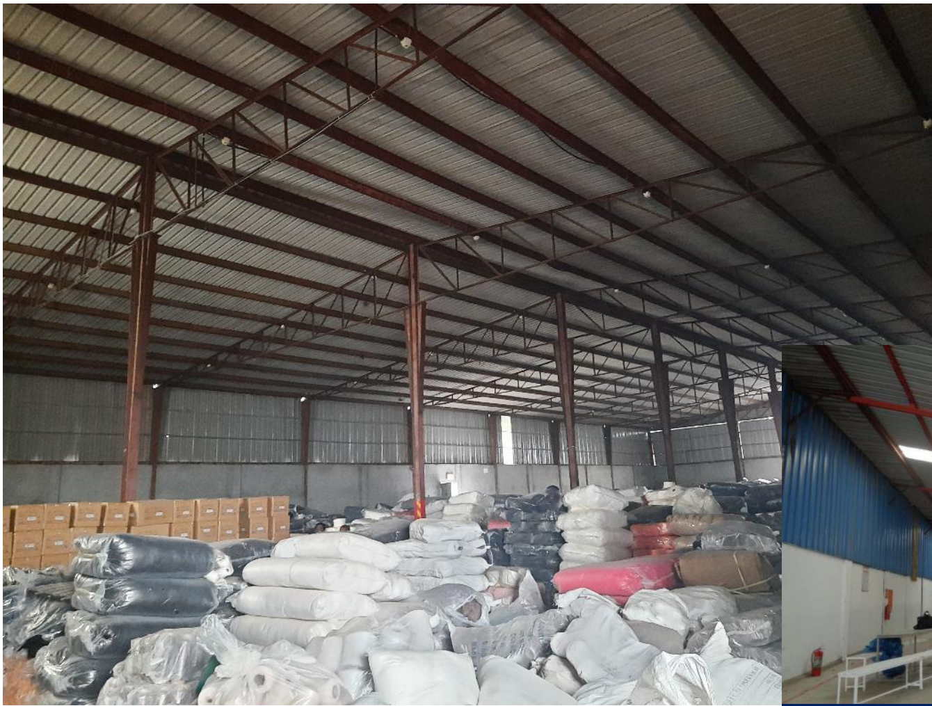
No roof bracing/compression member
