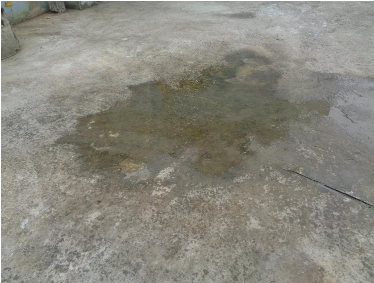
Water stagnant on roof slab
