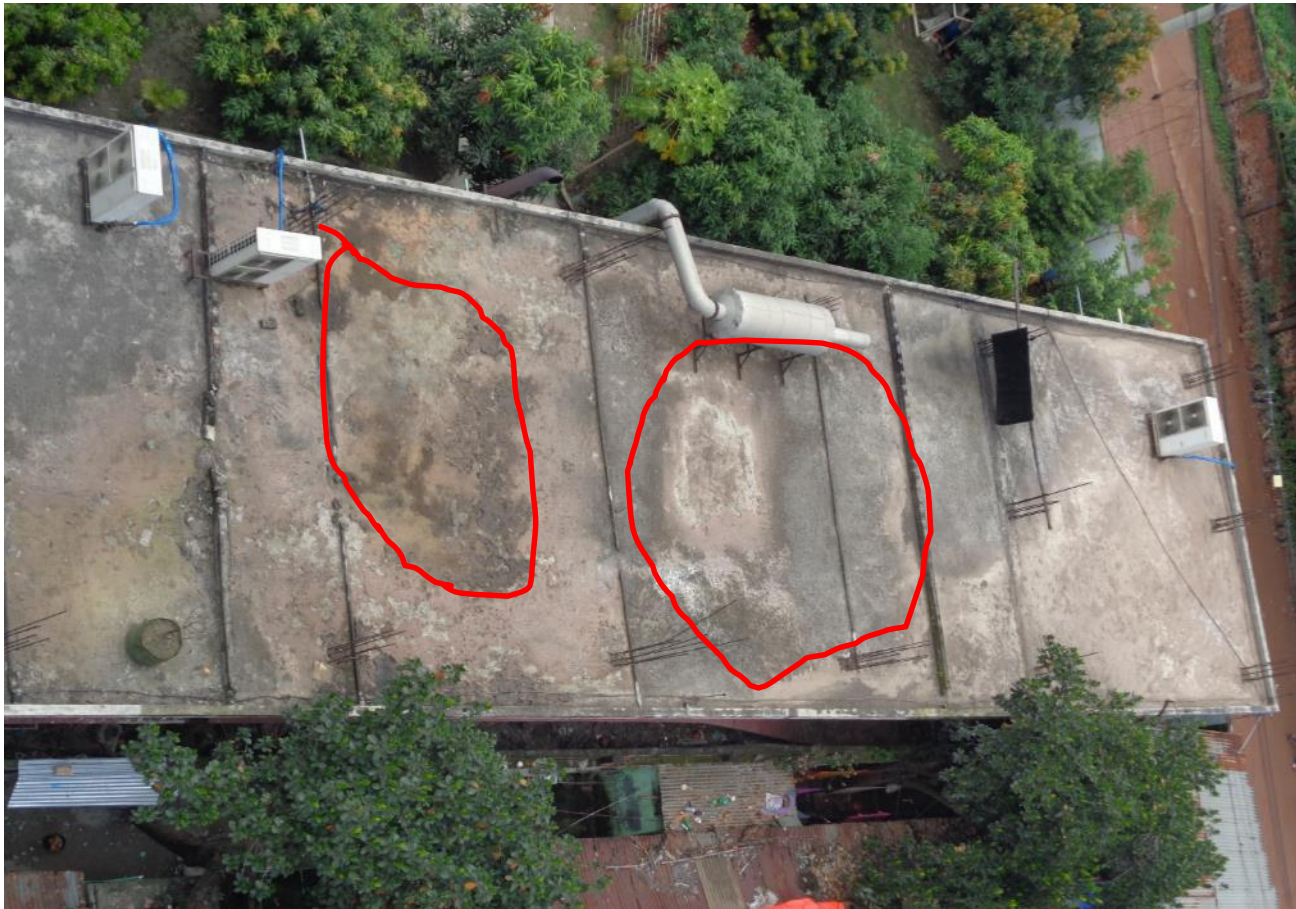
Water stagnant on roof slab
