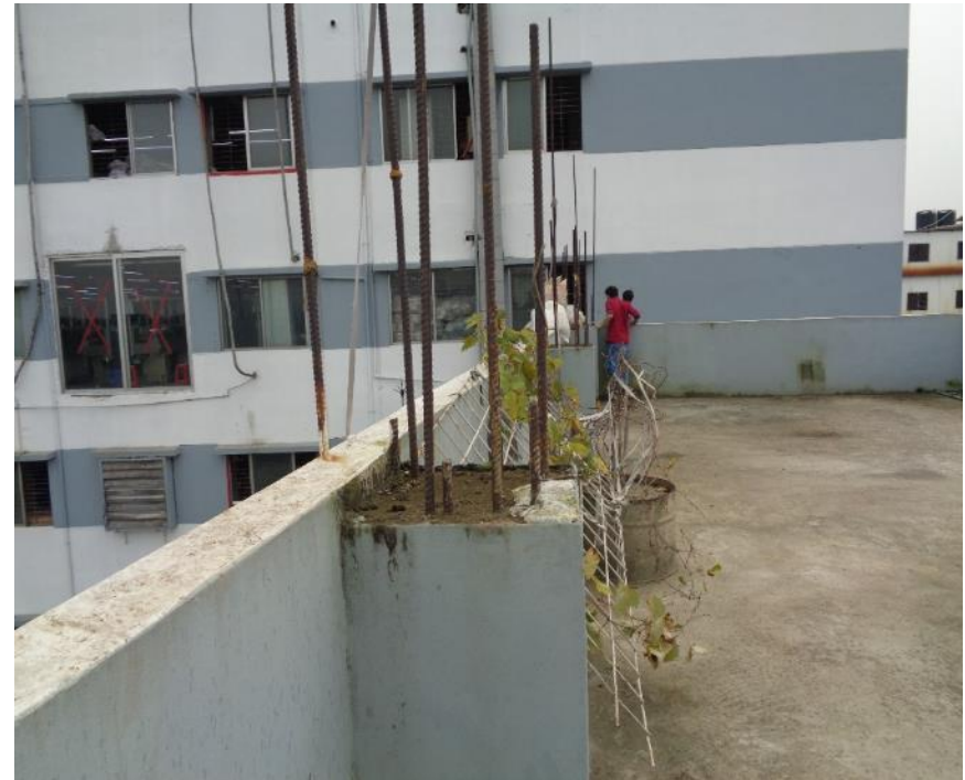
Exposed reinforcement left at roof
