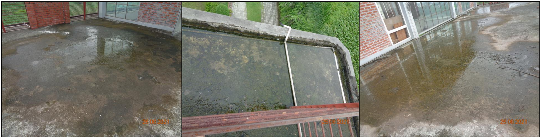
Water ponding at roof
