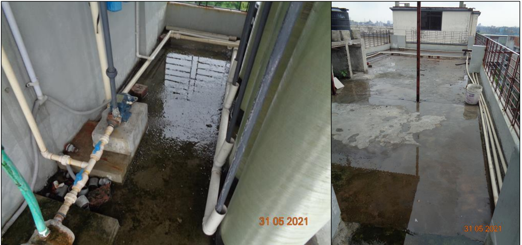
Water ponding at roof
