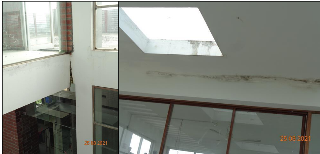
Dampness in Beam-Column & slab due to water ponding
