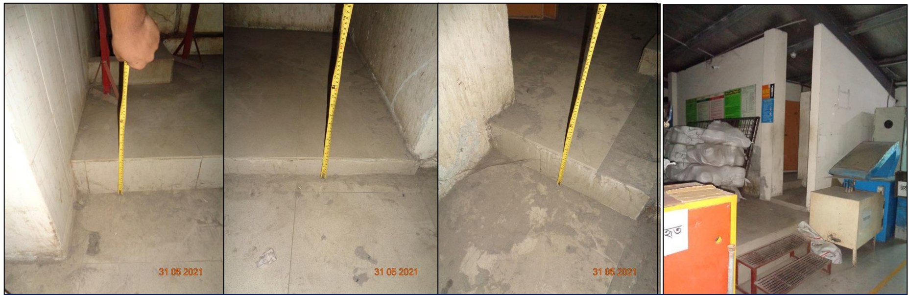
Build-up found at toile block area.
