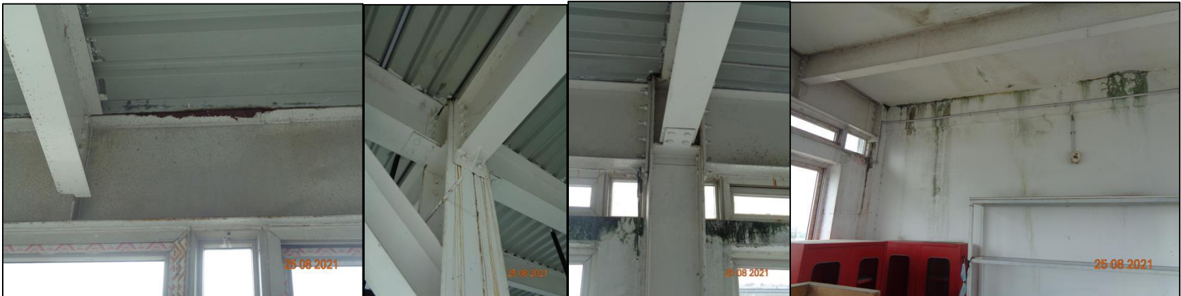
Due to the water ponding at roof, dampness and corrosion found in deck slab & steel sections
