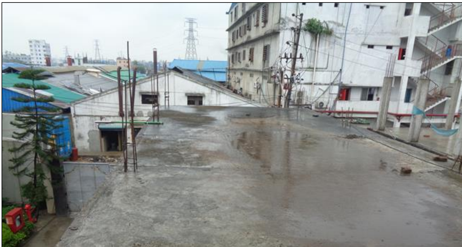
Water ponding at roof
