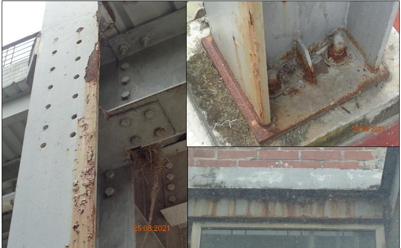
Corrosion in steel column
