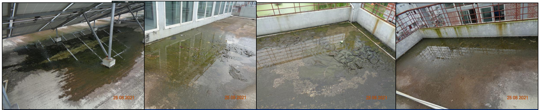
Water ponding at roof due to lack of proper drainage system & inadequate slope
