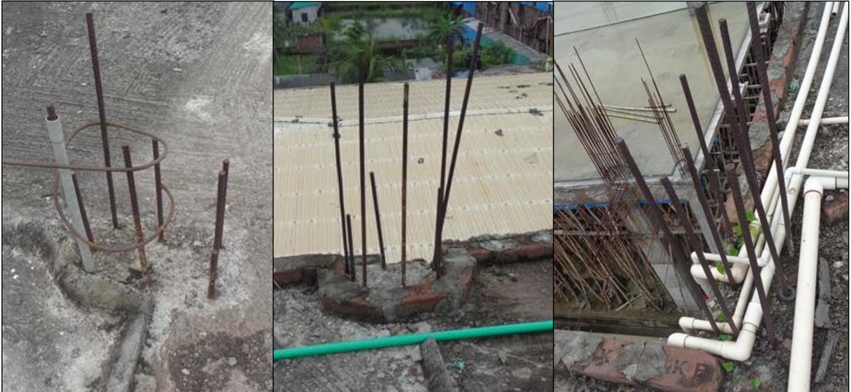
Exposed rebar of Column
