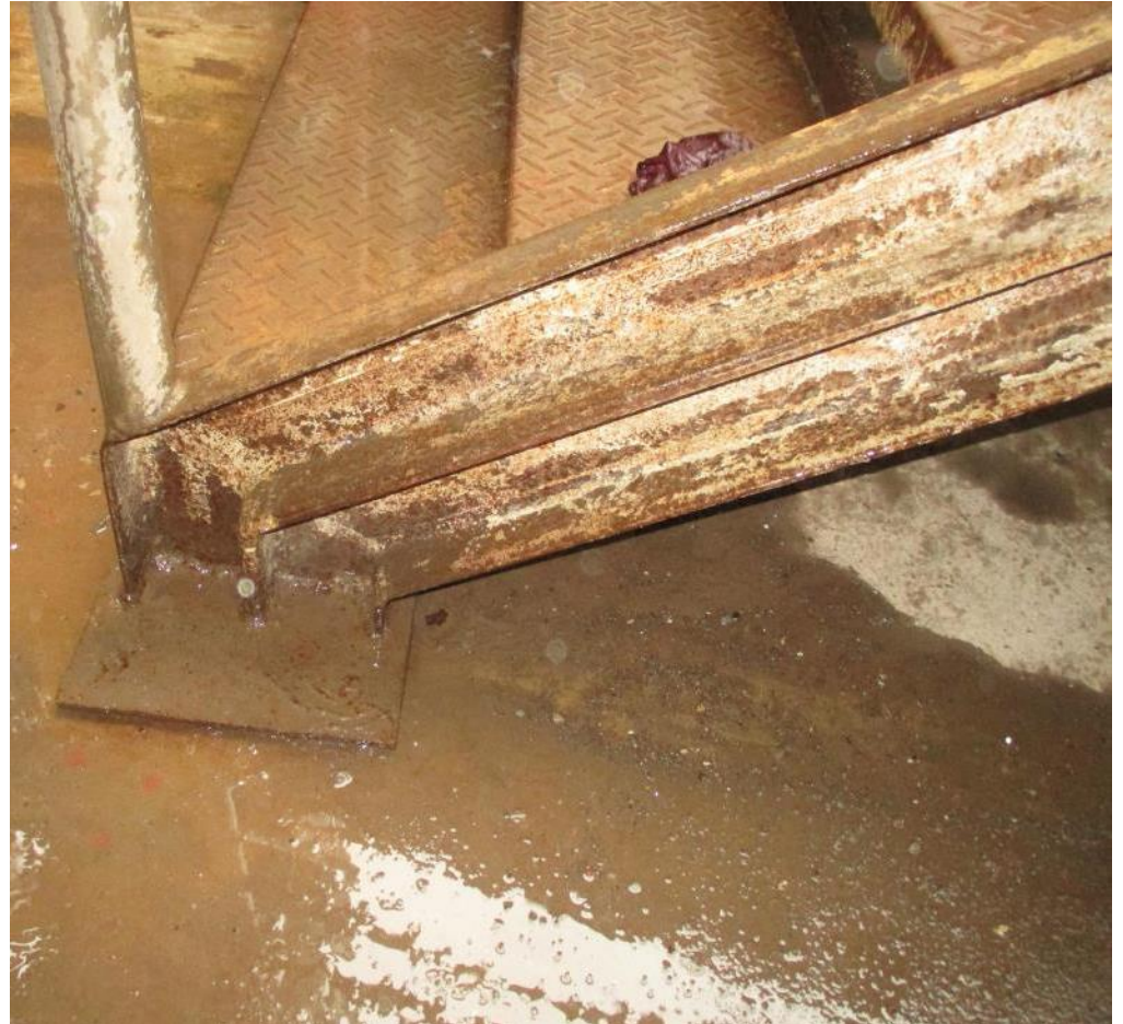
Corrosion found in steel stair
