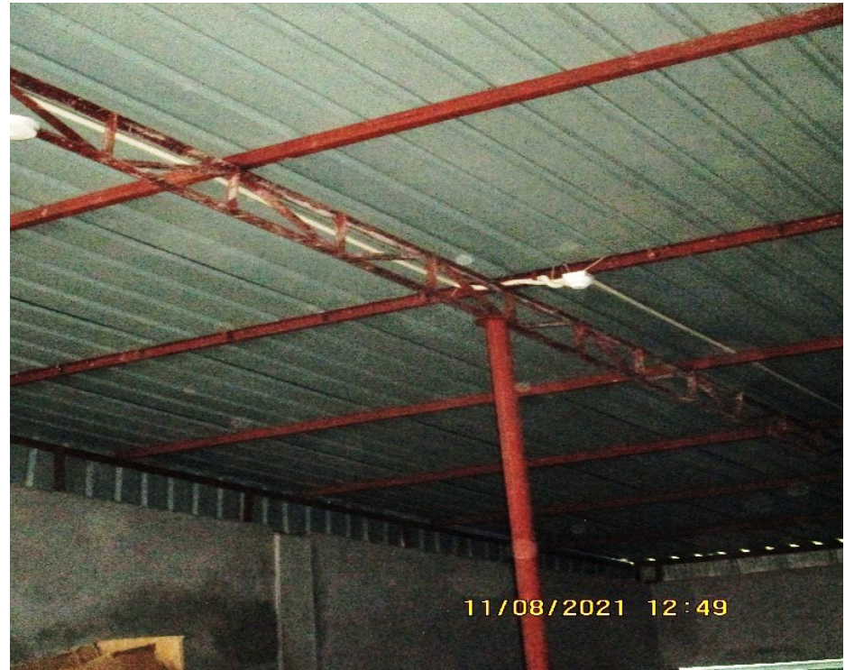
Apparently inadequate structural members
