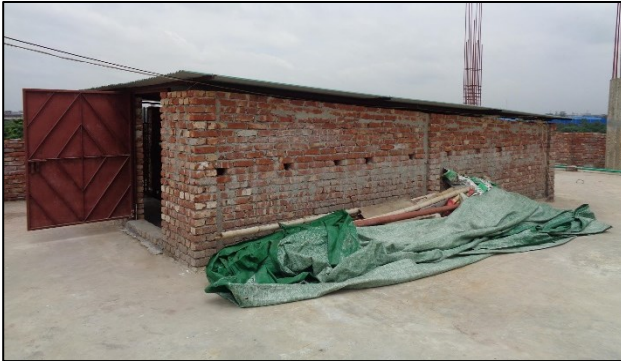
Tin roof on the existing staircase with poor anchorage
