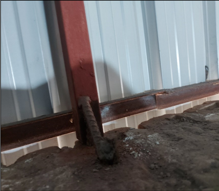
Poor connection details
