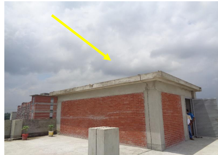
No overhead RC water tank on staircase roof.
