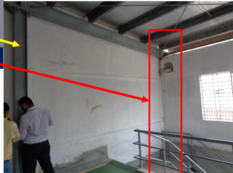
Column found at different position
