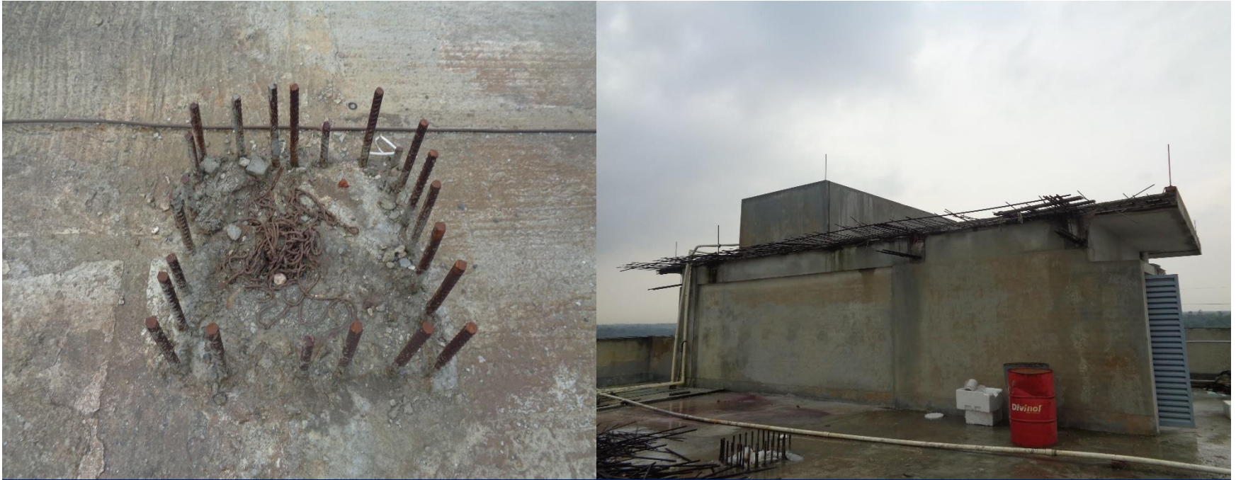
Exposed reinforcement left at roof level
