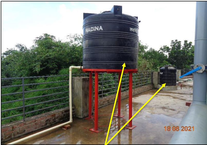
2 nos. Plastic Water Tank on roof top slab (Capacity- 2000 & 1000 Liter)
