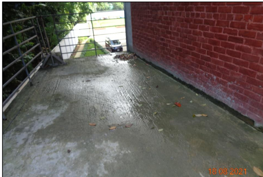
Water ponding on 1 st Floor Open to Sky Area
