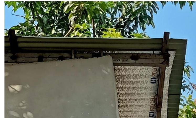
Non engineered connections (GF roof-East side)
