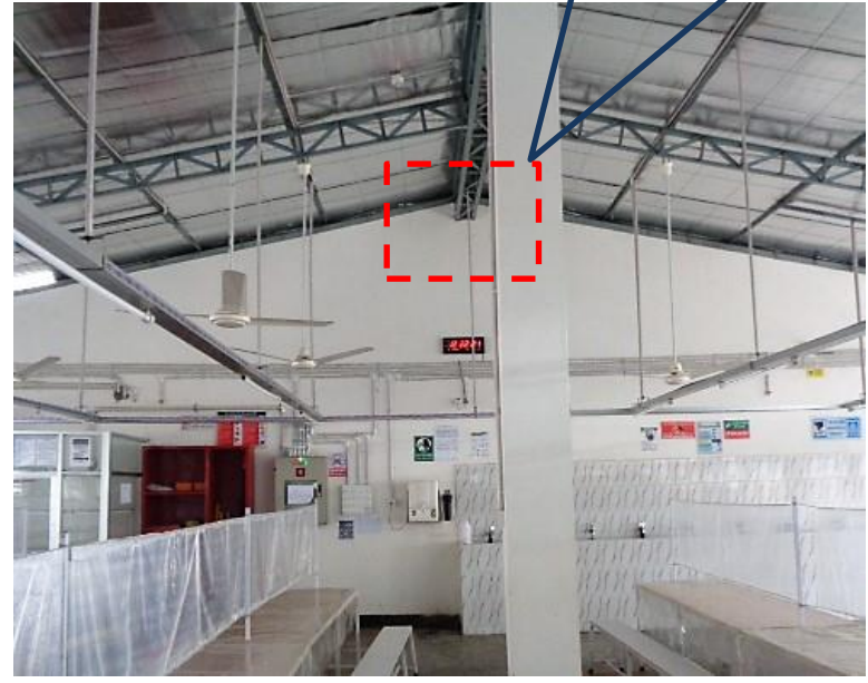
Two buildings are found structurally connected.
