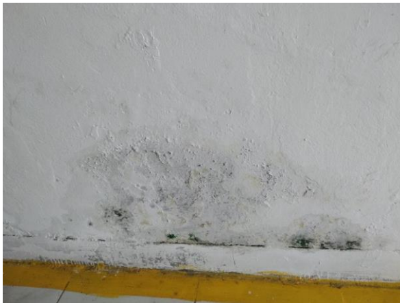
Dampness was found on the wall of toilet zone.
