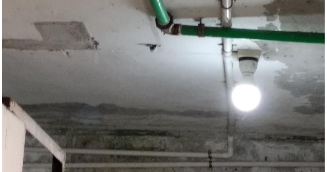
Dampness was found on slab at several locations.
