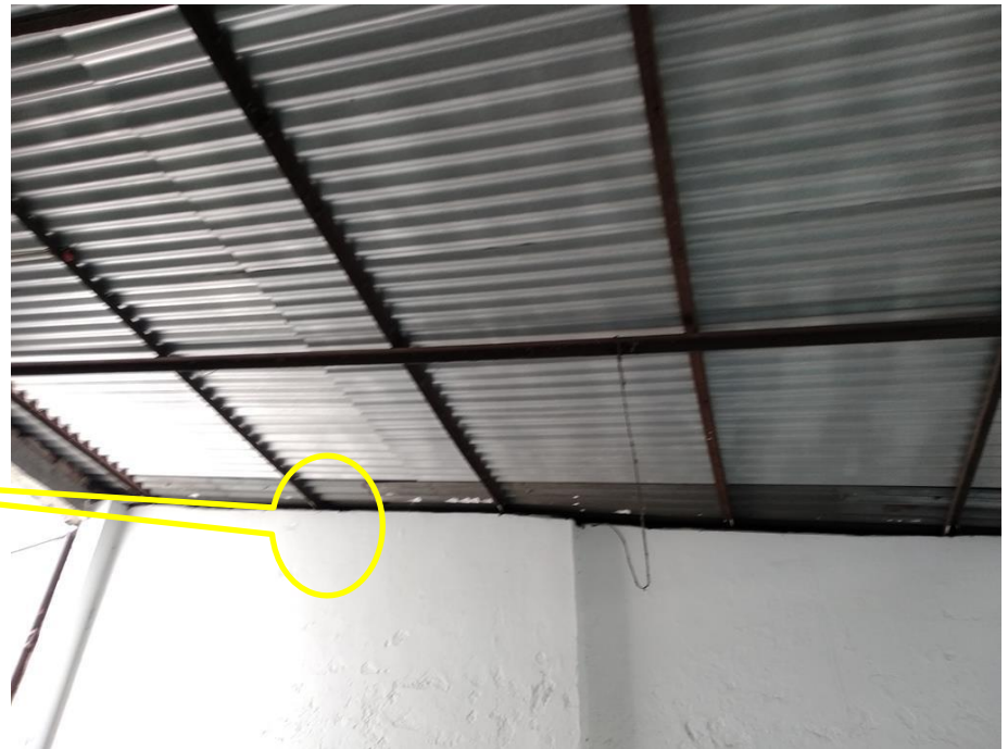
Inadequate structural members
