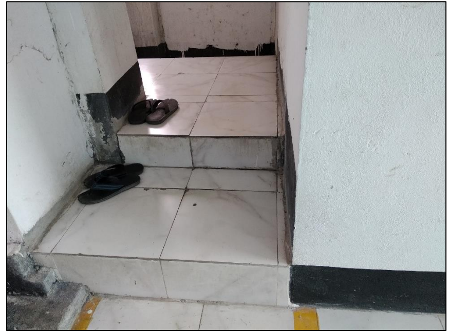
Build-up in toilet area
