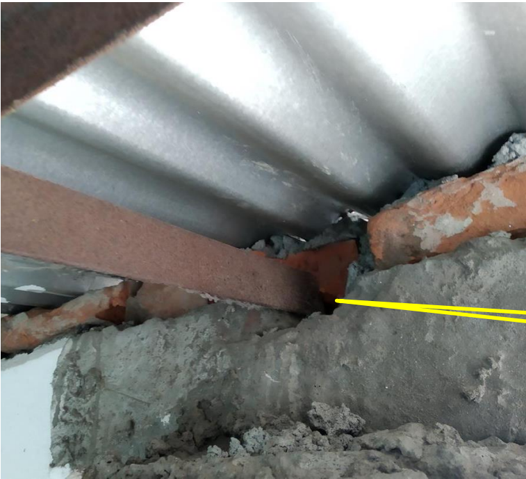
Poor connection details
