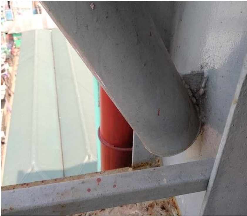
Poor connection of bracing
