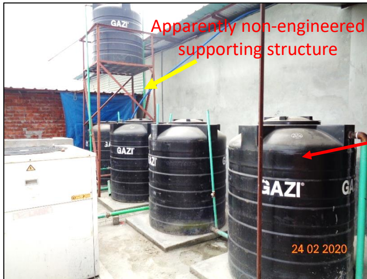
Undocumented 4 nos 1000 Ltr and 1 no 750 Ltr water Tank
