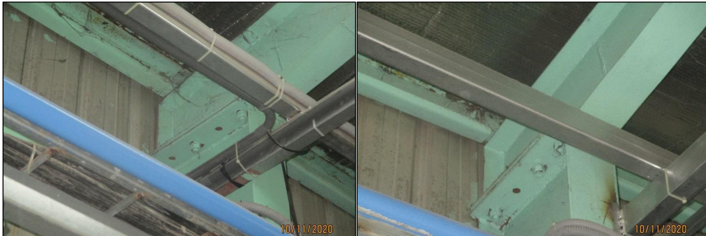
Bolt missing observed in several locations.
