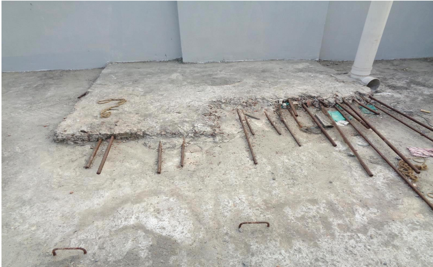
Exposed reinforcement at roof level
