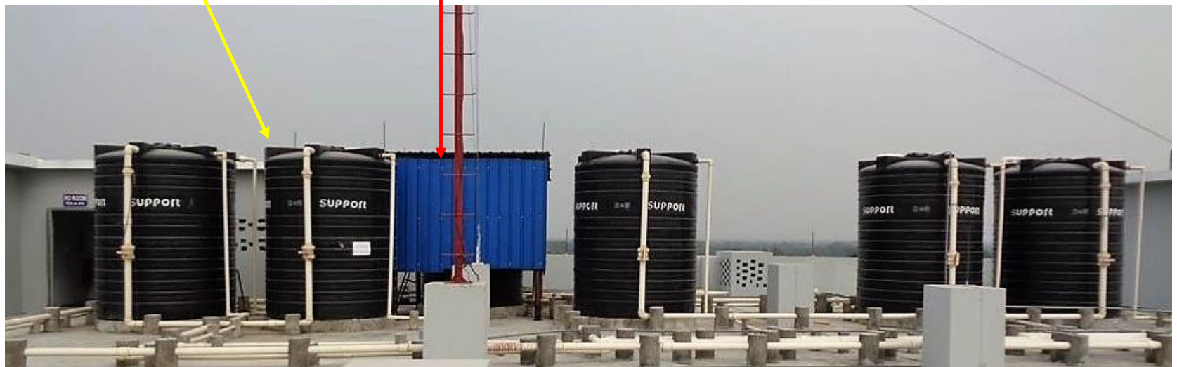
Plastic water tanks on roof top
