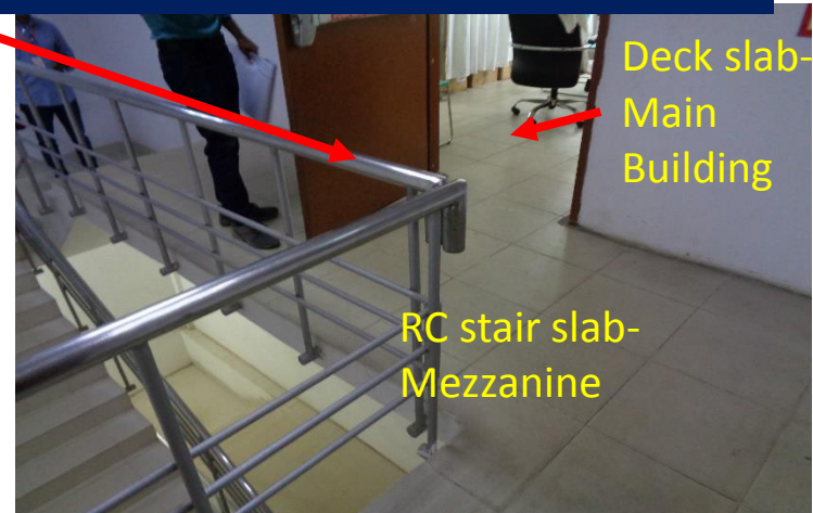
No separation was visible between RC and Deck slab
