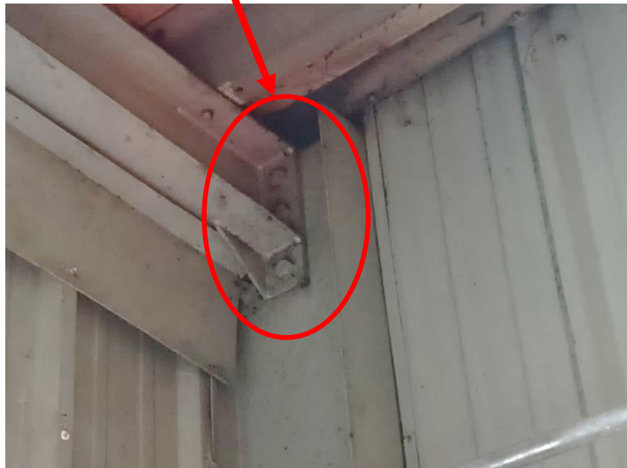
6-Bolts found physically
