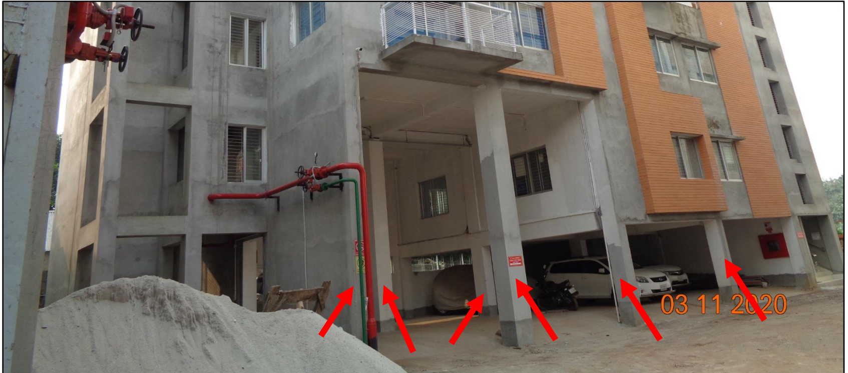
Columns having no barrier/protection at ground floor
