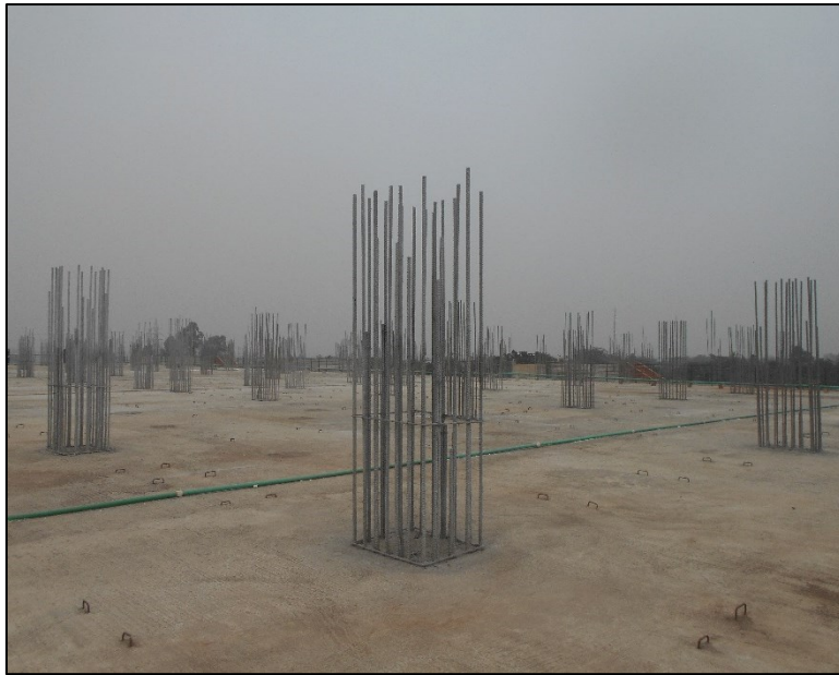
Exposed rebar on roof top
