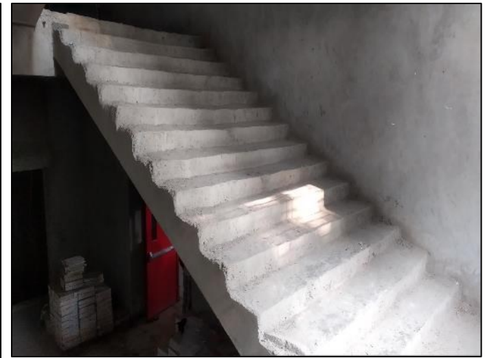
Railing missing on stair
