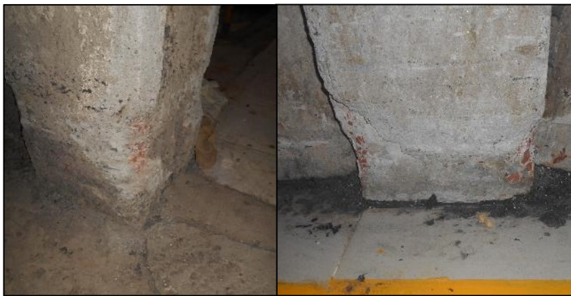
Damaged column of Shed C
