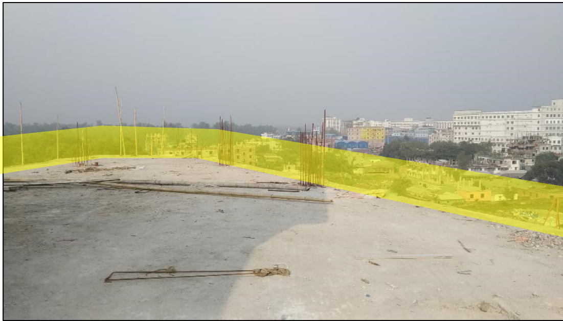
Roof without any parapet wall
