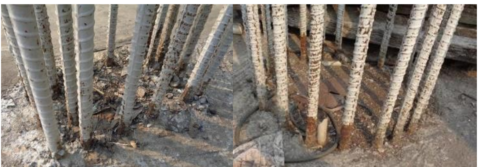
Corrosion in column re-bar
