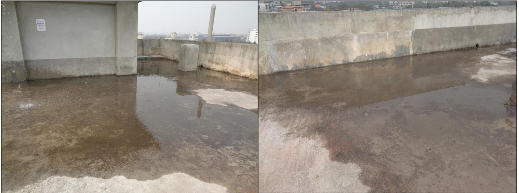
Water ponding on roof slab
