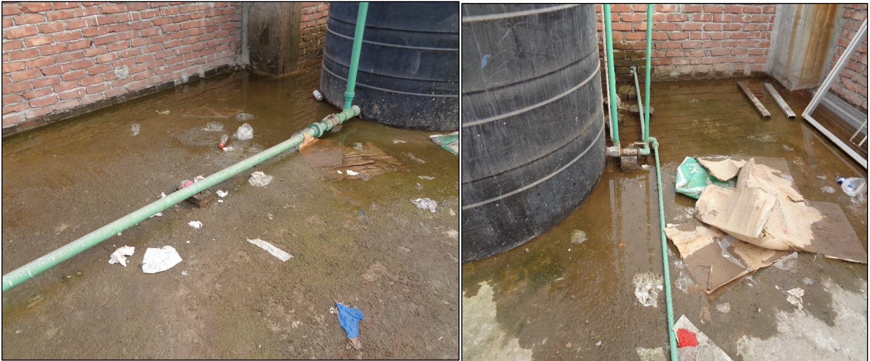
Water ponding on roof slab
