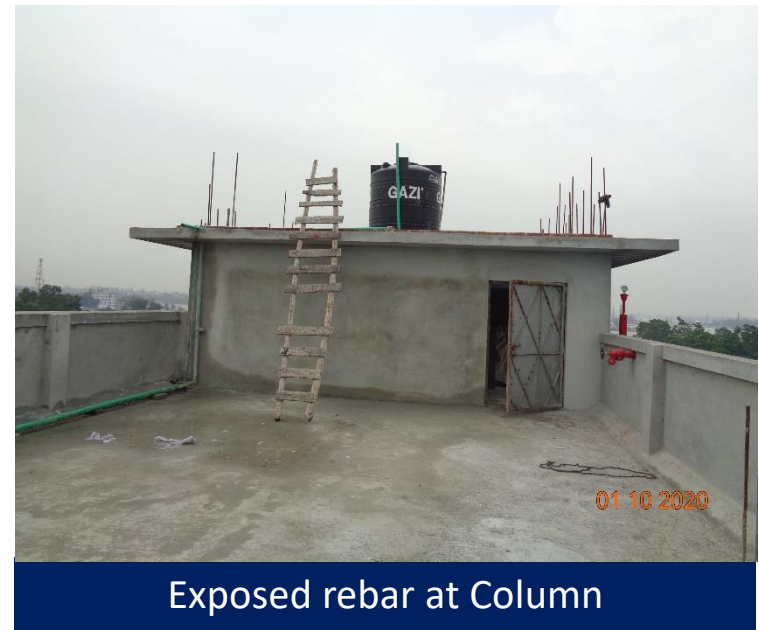
Exposed rebar at Column
