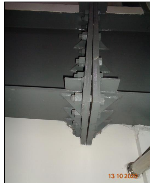
Connection Gap in Rafter
