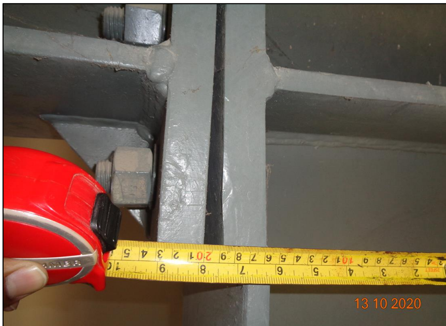
Gap observed in Beam- Column connection
