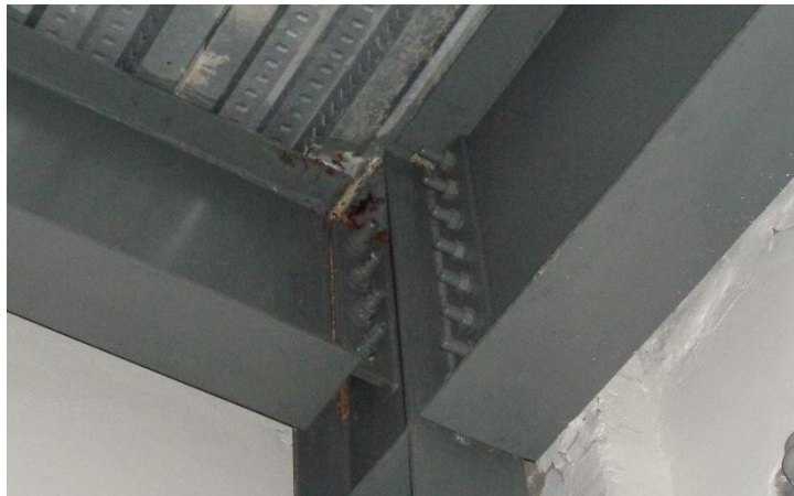
Corrosion in steel beam
