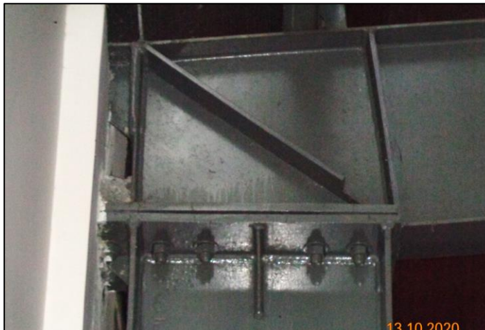
Gap observed in Rafter-Column connection
