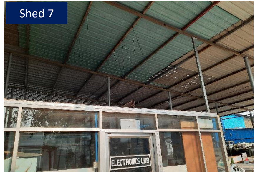
Inadequate structural members
