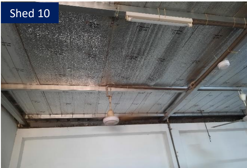
Inadequate structural members
