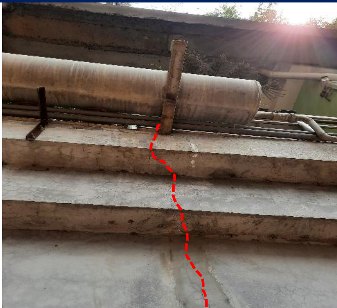
Formation of vertical cracks
