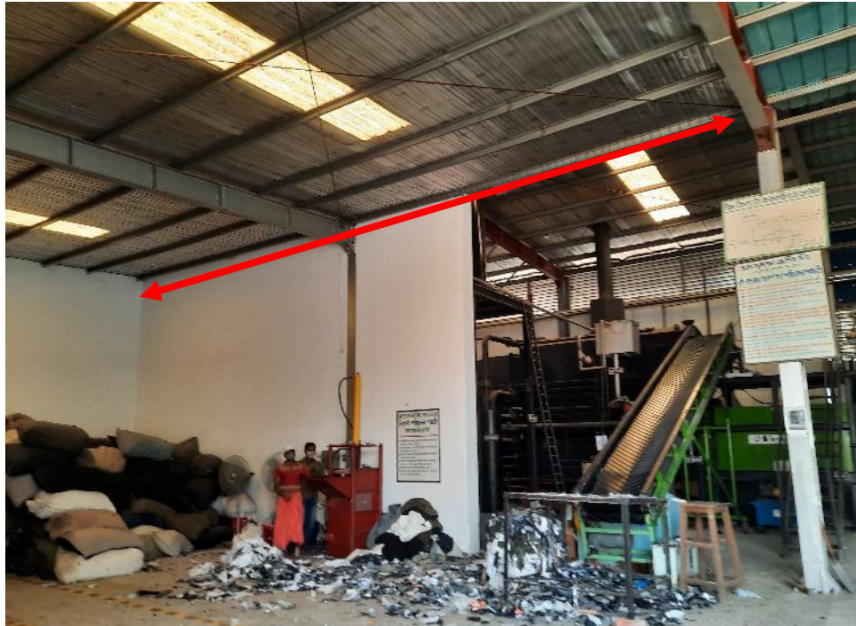
Missing compression member in long direction
