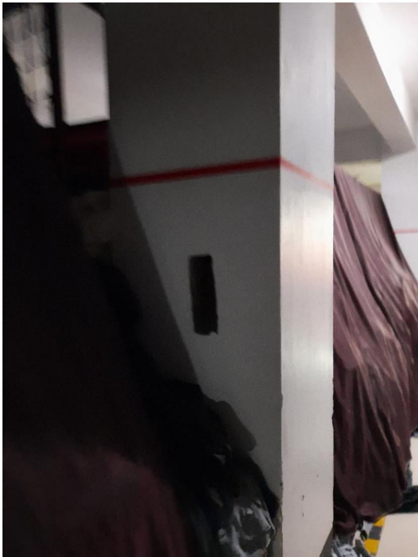
Electrical cable hole
