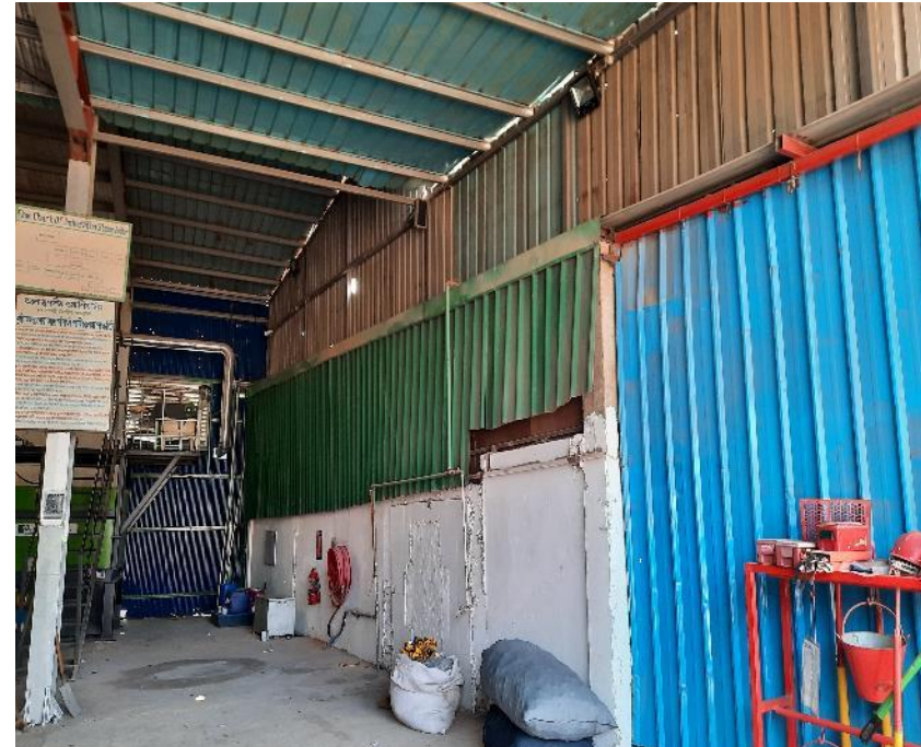
Cantilever portion of the shed not adequately connected
