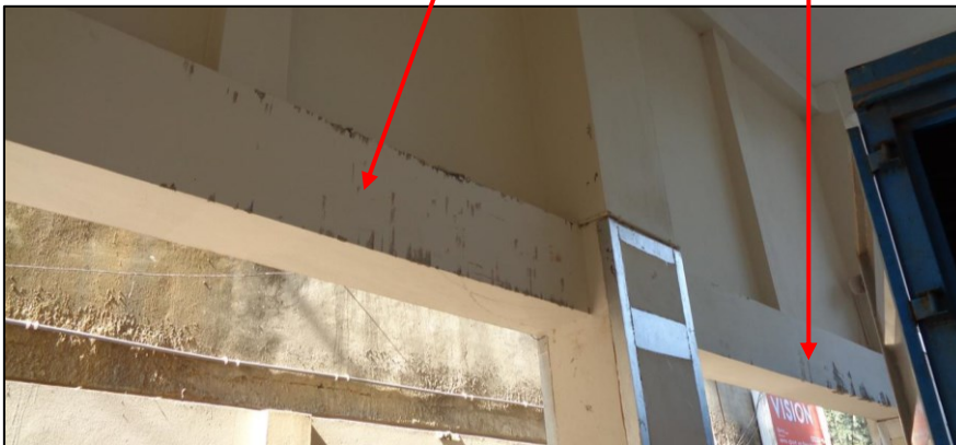
Partial damaged beam
