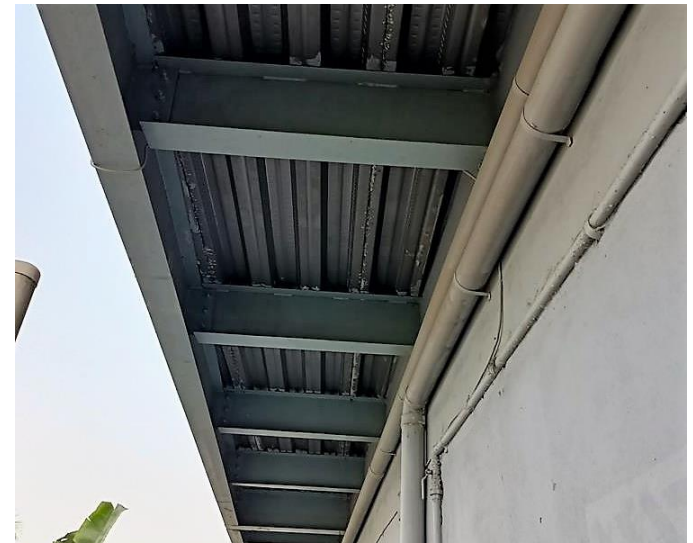
Connection details was not provided for the cantilever areas.
