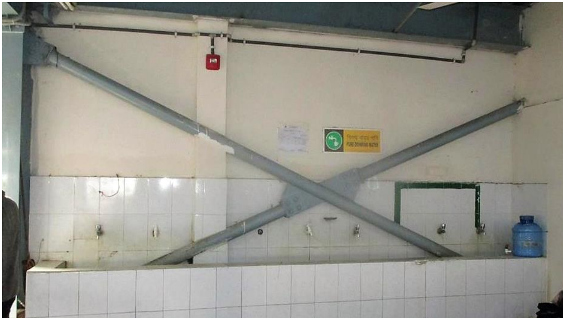
No connection details of the vertical bracings was provided in the as-built structural drawing of Shed-3.
