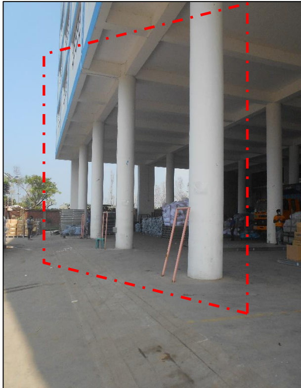
Insufficient column guard on ground floor exterior column only
