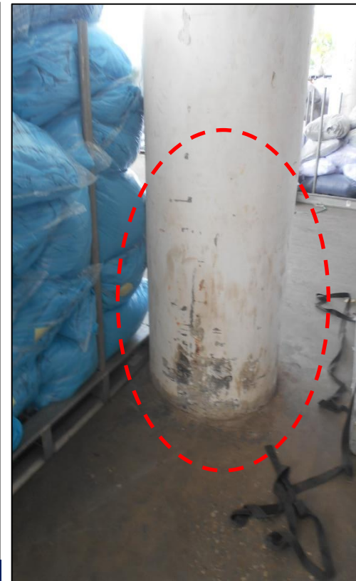
Sign of impact on ground floor internal column
