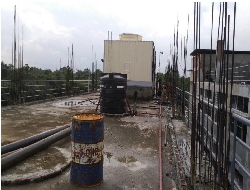
Exposed rebar at Column
