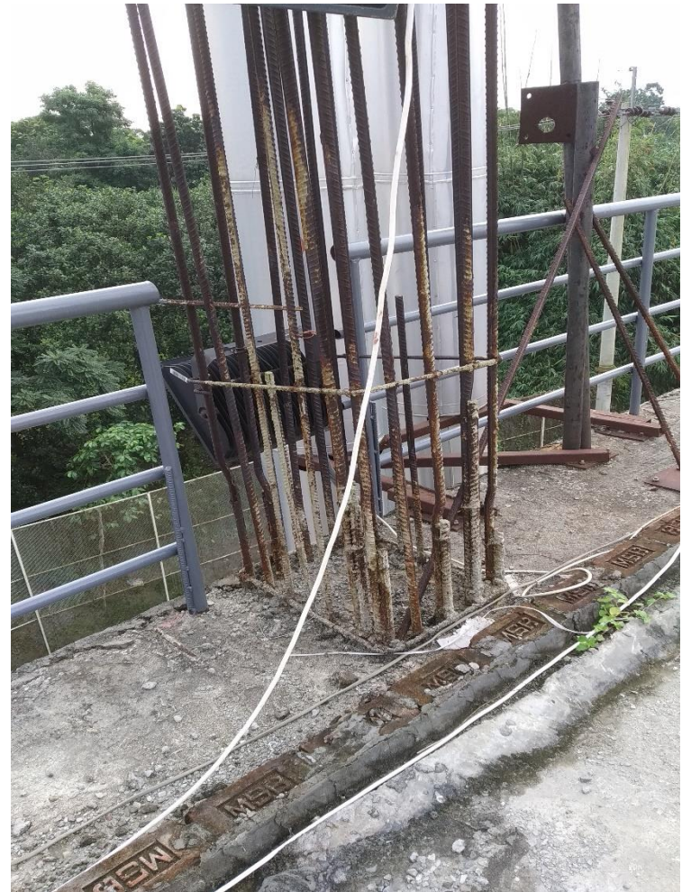
Exposed rebar at Column
