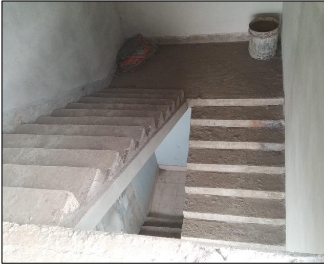
Railing is missing at staircase
