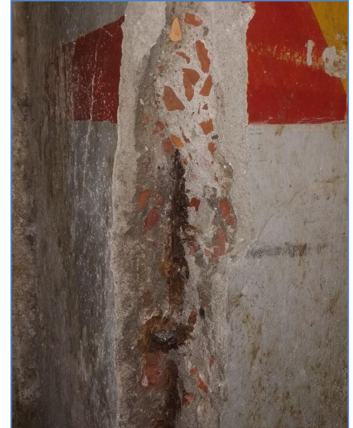
Crack extended to rebars
