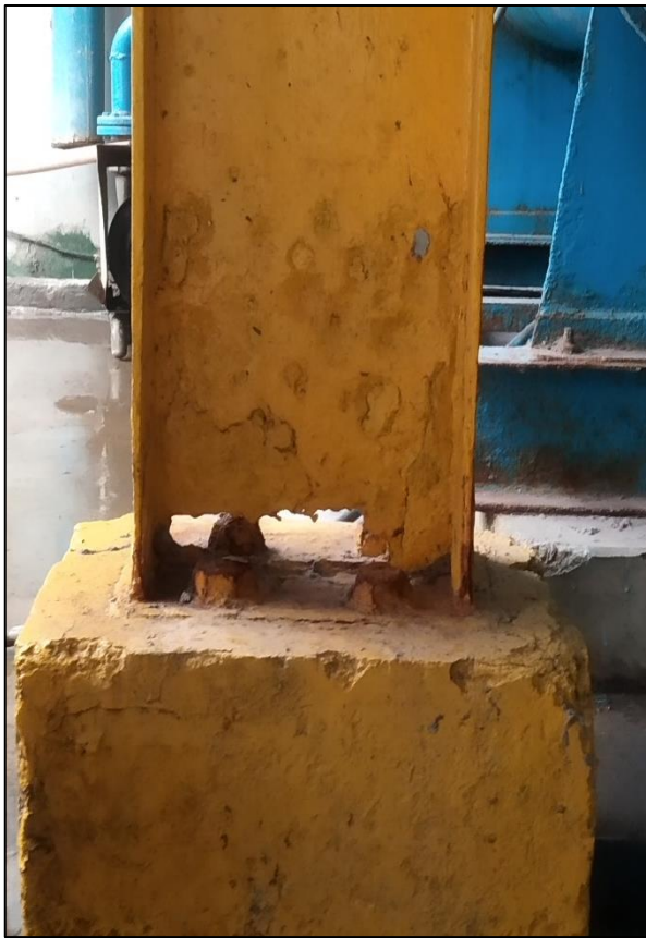
Corrosion damaged column
