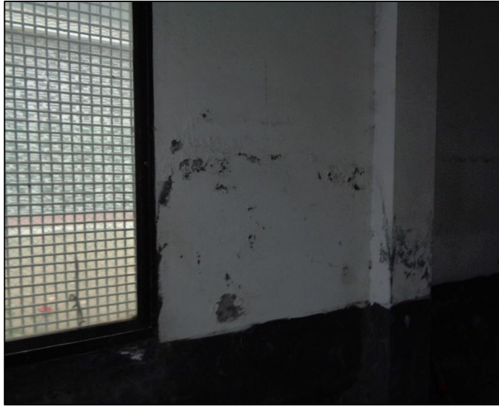
Dampness in wall
