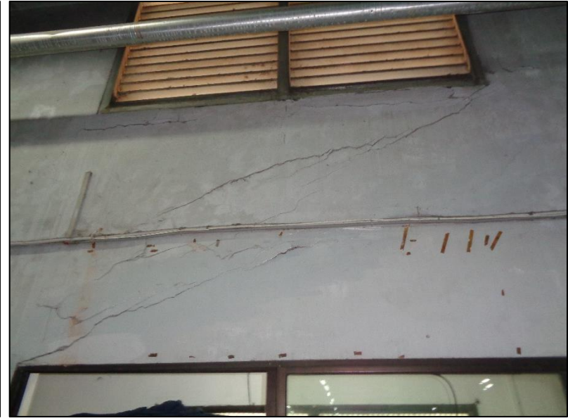
Crack in wall
