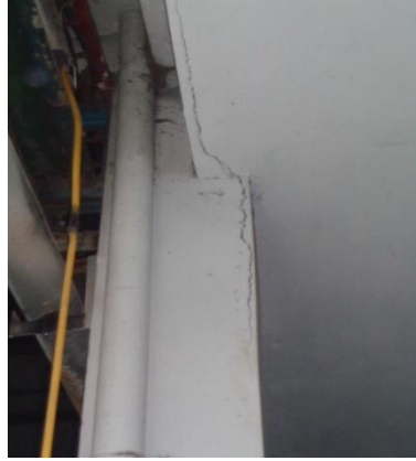
Slab of dyeing office appears to be connected with column of dyeing shed (part-A)
