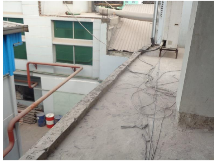
Cantilever portion has no railing
