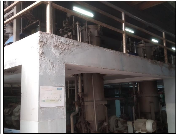
Dampness in column
