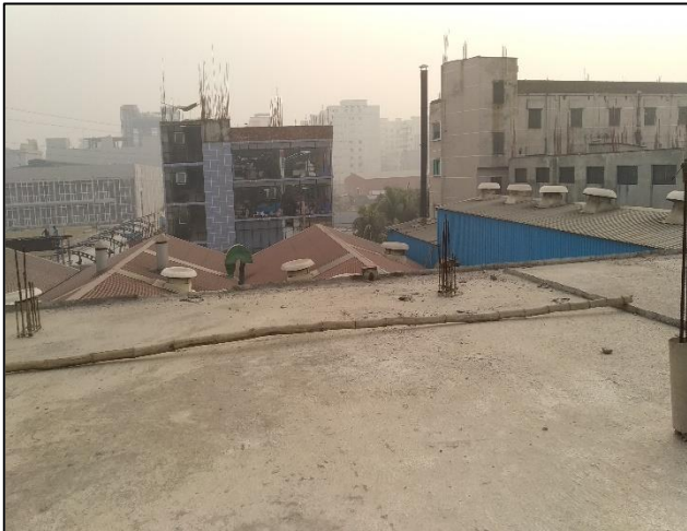
Roof has no parapet wall
