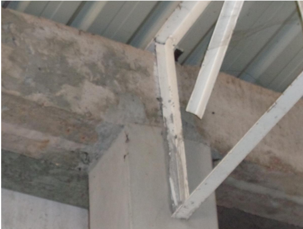
Roof framing in the storage shed utilizing truss framing was poorly build and employed questionable framing methods
