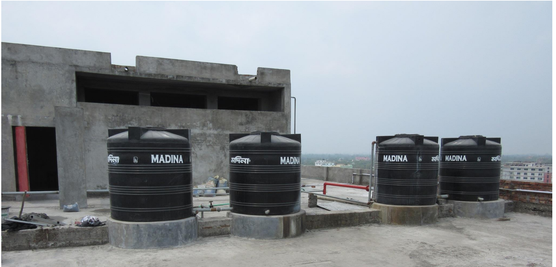
Water tanks are positioned in one line
