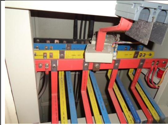
Busbar of distribution panel.
