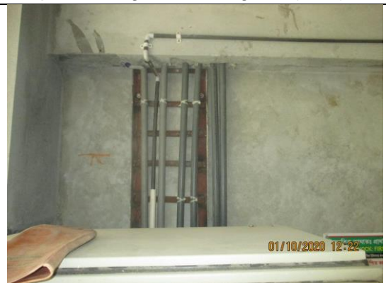
Typical cable entry system into electrical panel in production floors.
