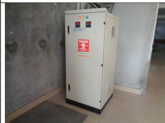
Typical electrical distribution panel.
